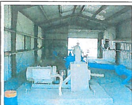
October 13, 2008 Generator on the geothermal hydro
