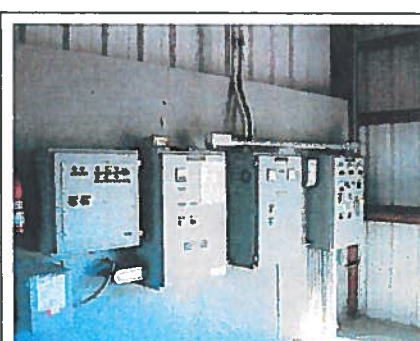
October 13, 2008 Electrical controls at the geothermal hydro
