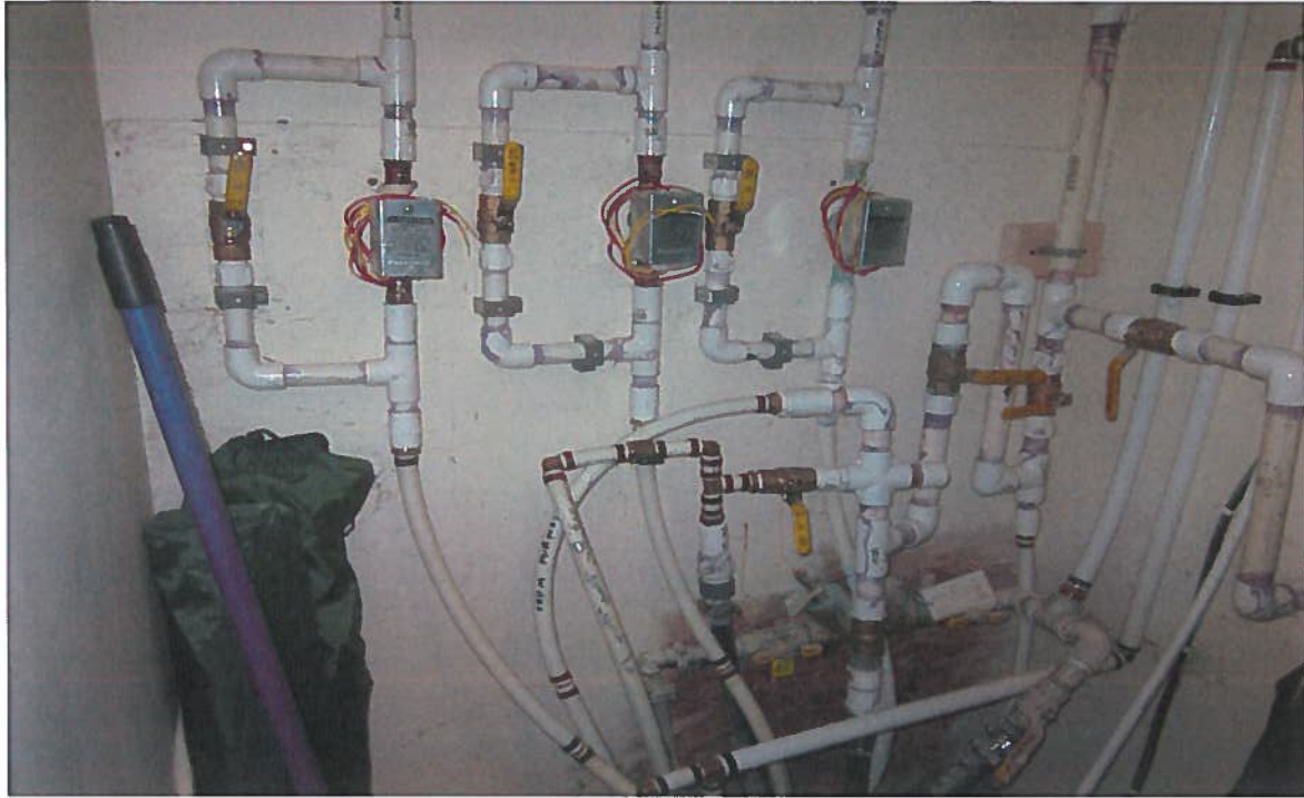
Geothermal system piping in the garage.
