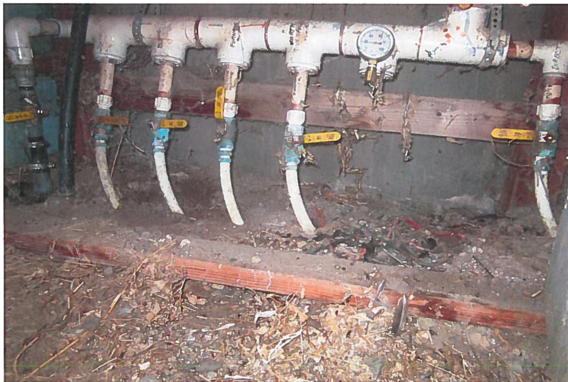
Inside the control box located by the bridge. Hot water is piped to different zones.
