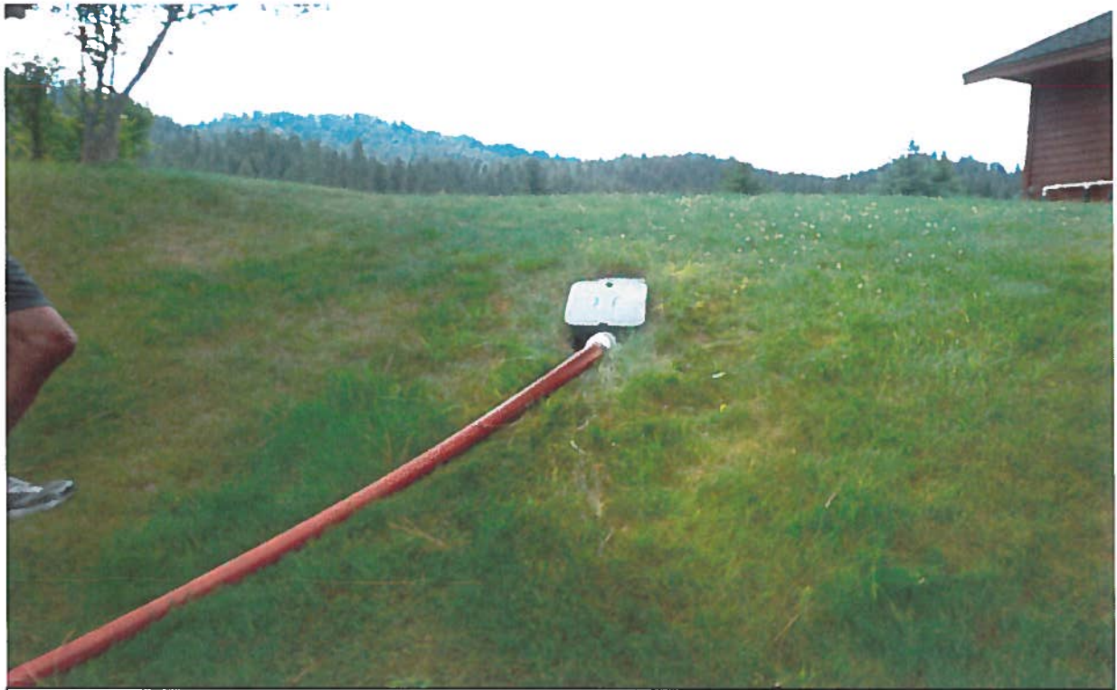
View southeasterly of the point of connection of the 2" flexible hose discharge line to the buried 4" PVC irrigation main line.
