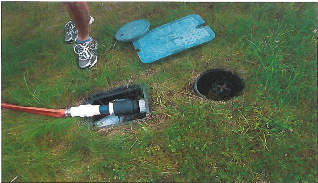
View of the 2" flexible hose discharge line connected to the 4" PVC buried irrigation main line. The hand operated gate valve controls the flow to the field hand line irrigation system or to the lawn and landscaping pressurized irrigation system.
