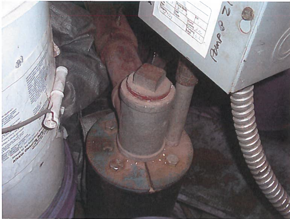
63-11764 Exam 8/27/2012: POD well inside pump house.
