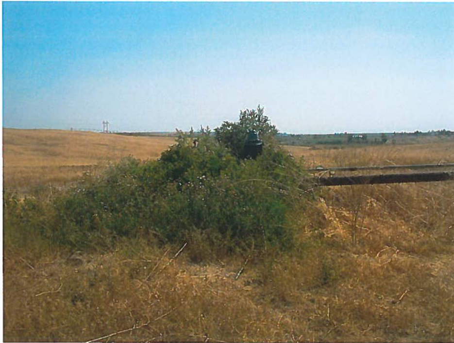
63-31982 Exam 8/30/2012: Motor pumps water from buried storage tank facing south. 2 inch line from well to buried storage tank and 6 inch line from storage tank to 8 inch mainline. East side of pump house.
