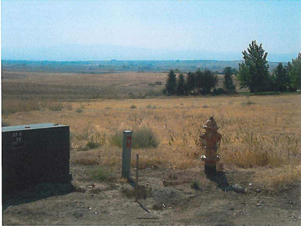
63-31982 Exam 8/30/2012: Initial fire hydrant off buried 8 inch mainline facing south. POD pump house in photo middle ground left of evergreen trees.
