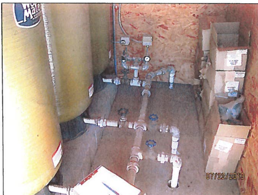
Figure 10: Well #5 pump house plumbing.
