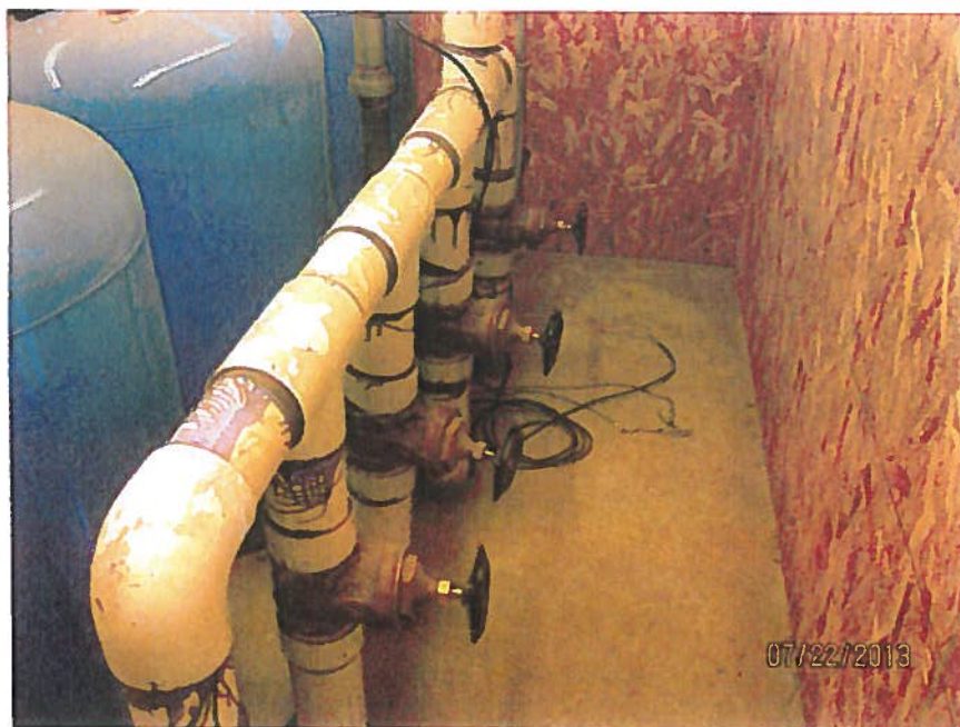
Figure 14: Well #7 pump house plumbing.
