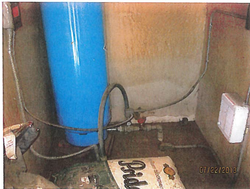
Figure 2: Well 1 pump house.
