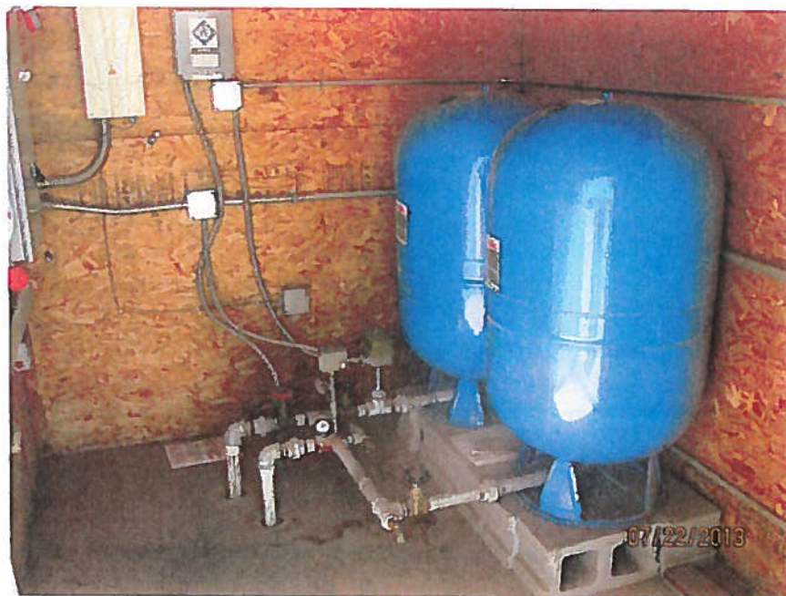
Figure 4: Well #2 pump house plumbing.
