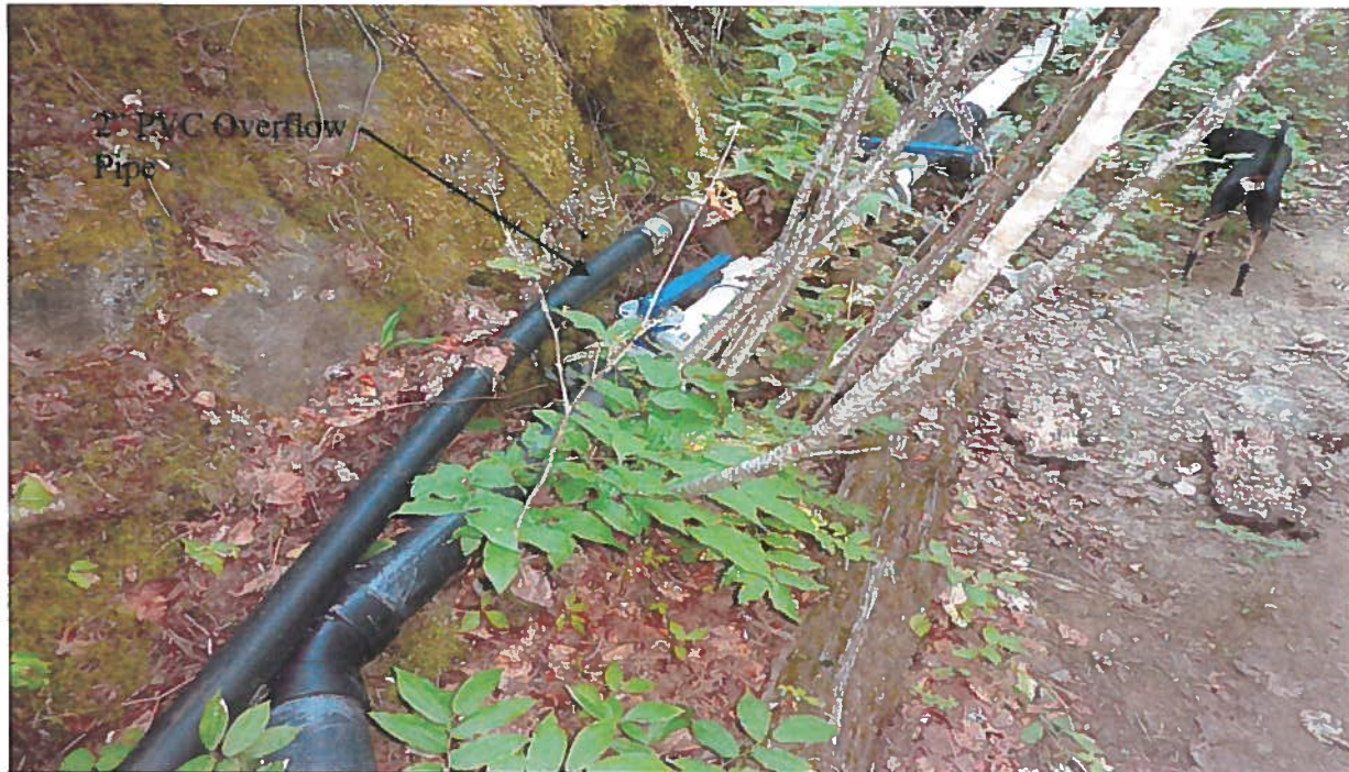
View of the 4" PVC supply line and a 2" PVC overflow pipe. The 2" PVC overflow pipe expands to 4" PVC prior to discharging to Little Elk Creek. The two valves on the 4" PVC supply line regulate the flow to the storage pond and the overflow pipe to Little Elk Creek.
