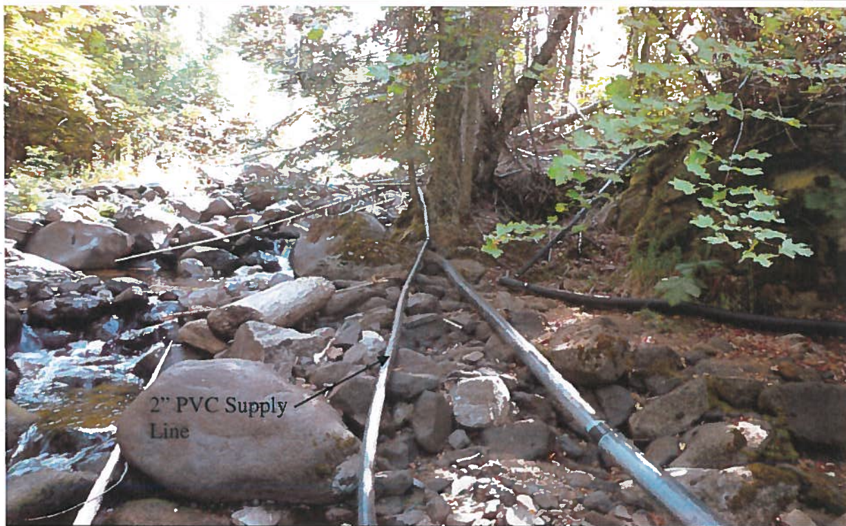
View upstream of Little Elk Creek of the 2" PVC supply line. Miscellaneous PVC pipe sections are scattered along the bank of Little Elk Creek.
