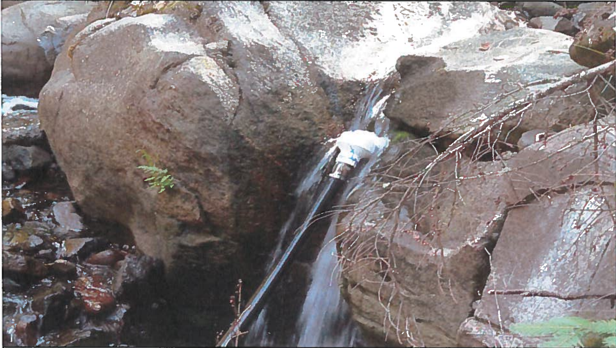
Point of Diversion: View of 2" PVC supply line with a 2" PVC reducer to capture water from Little Elk Creek.
