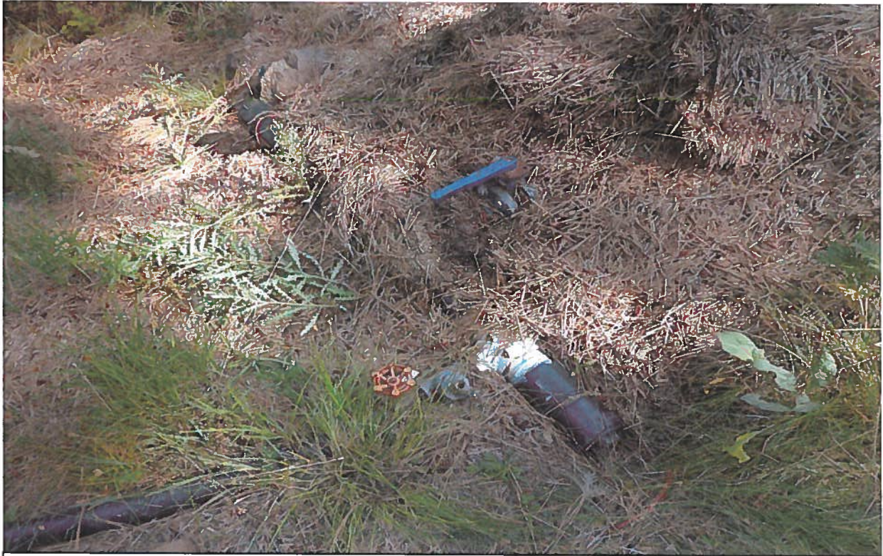
View of the 4" PVC discharge manifold located at the toe of the dam. The blue handled valve controls flow from the storage pond. The gold gate valve controls the flows to the irrigation system around the home.
