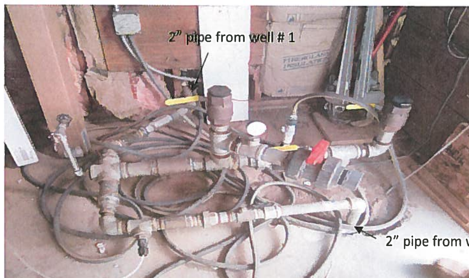
Interior of the cold water pump house. Pressure gauge indicated 52 psi.
