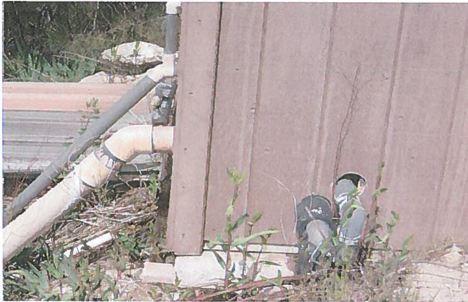
Water from the spring in the large pool pumped through 6" steel pipe in and out of lower pump house.
