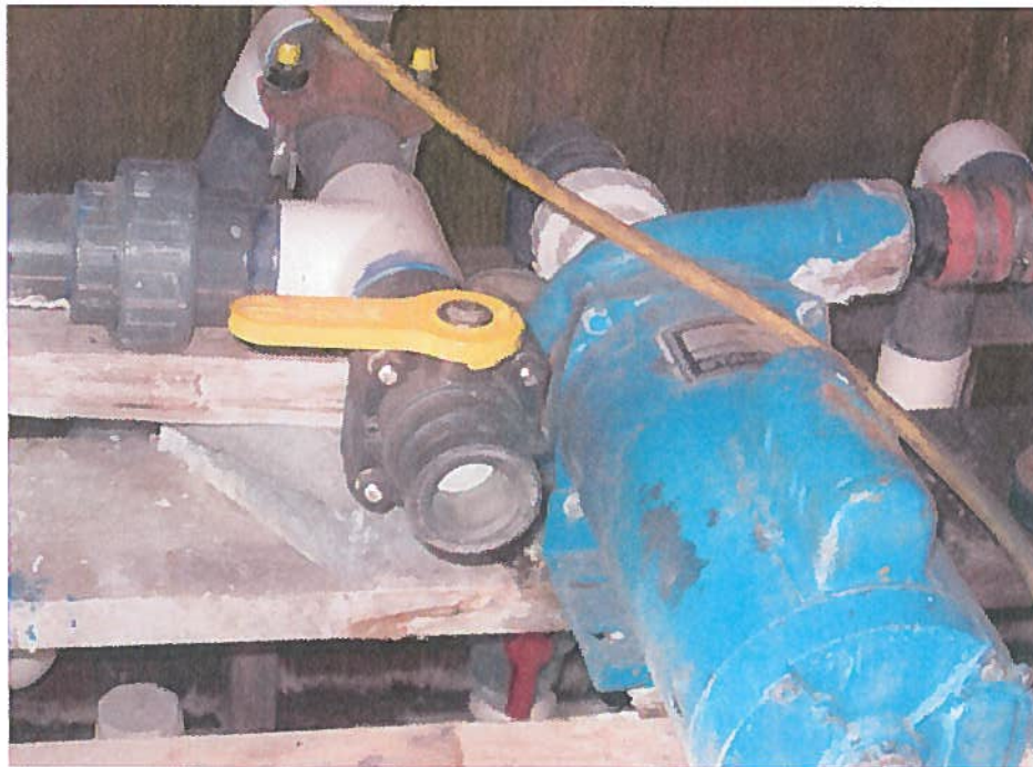
One of the 6 pumps inside the lower pump house.
