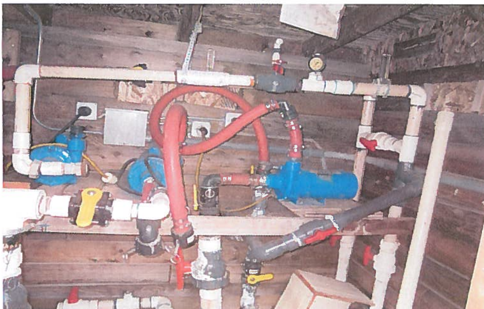
Interior of the upper pump house. Three Sta-rite 2.5 hp pumps seen.
