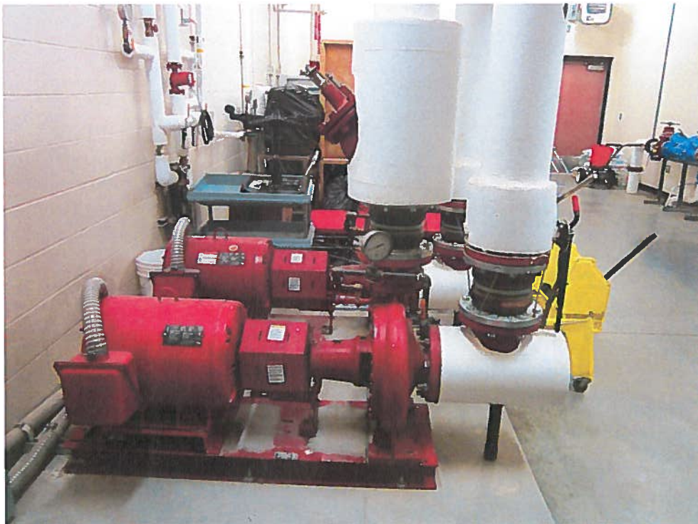
Figure 3: Pumps on internal distribution system
