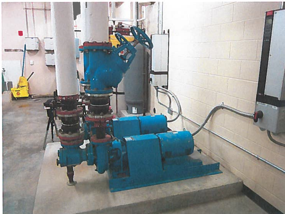
Figure 3: Pumps for distribution system
