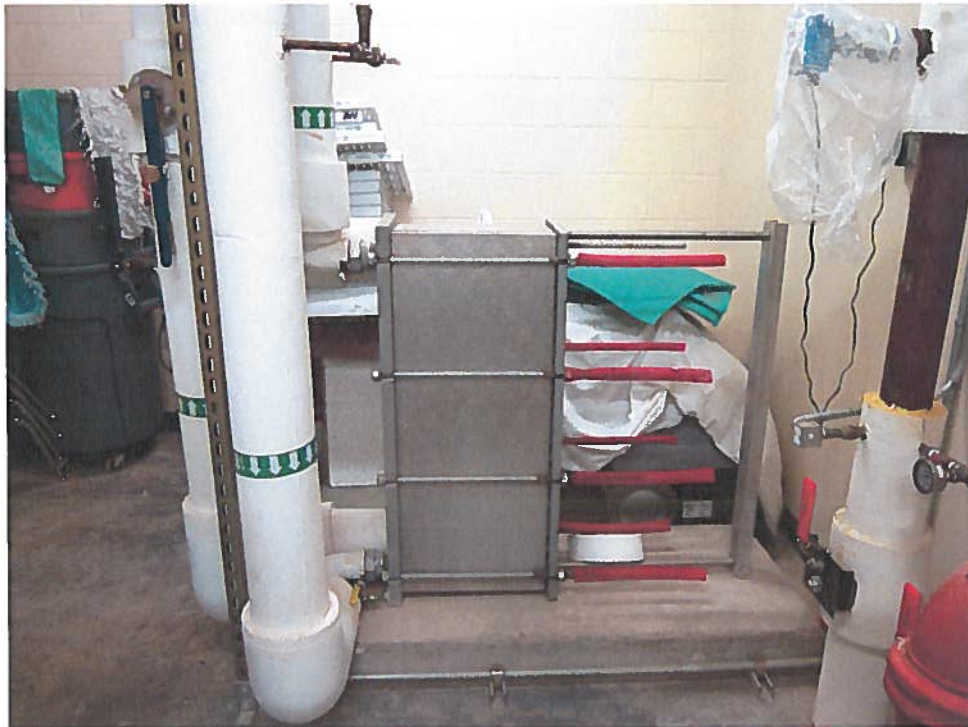
Figure 2: Heat exchanger and meter (covered with plastic bag)
