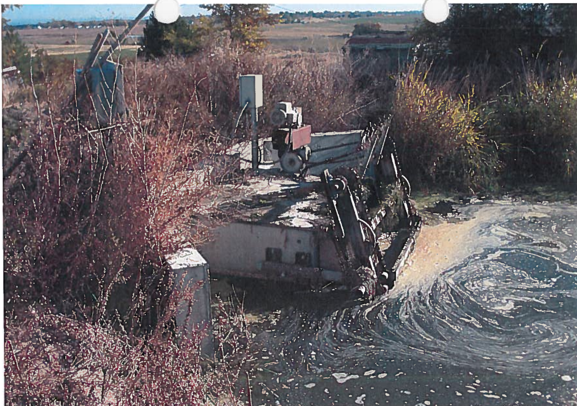
POD – Trash rack and penstock inlet
