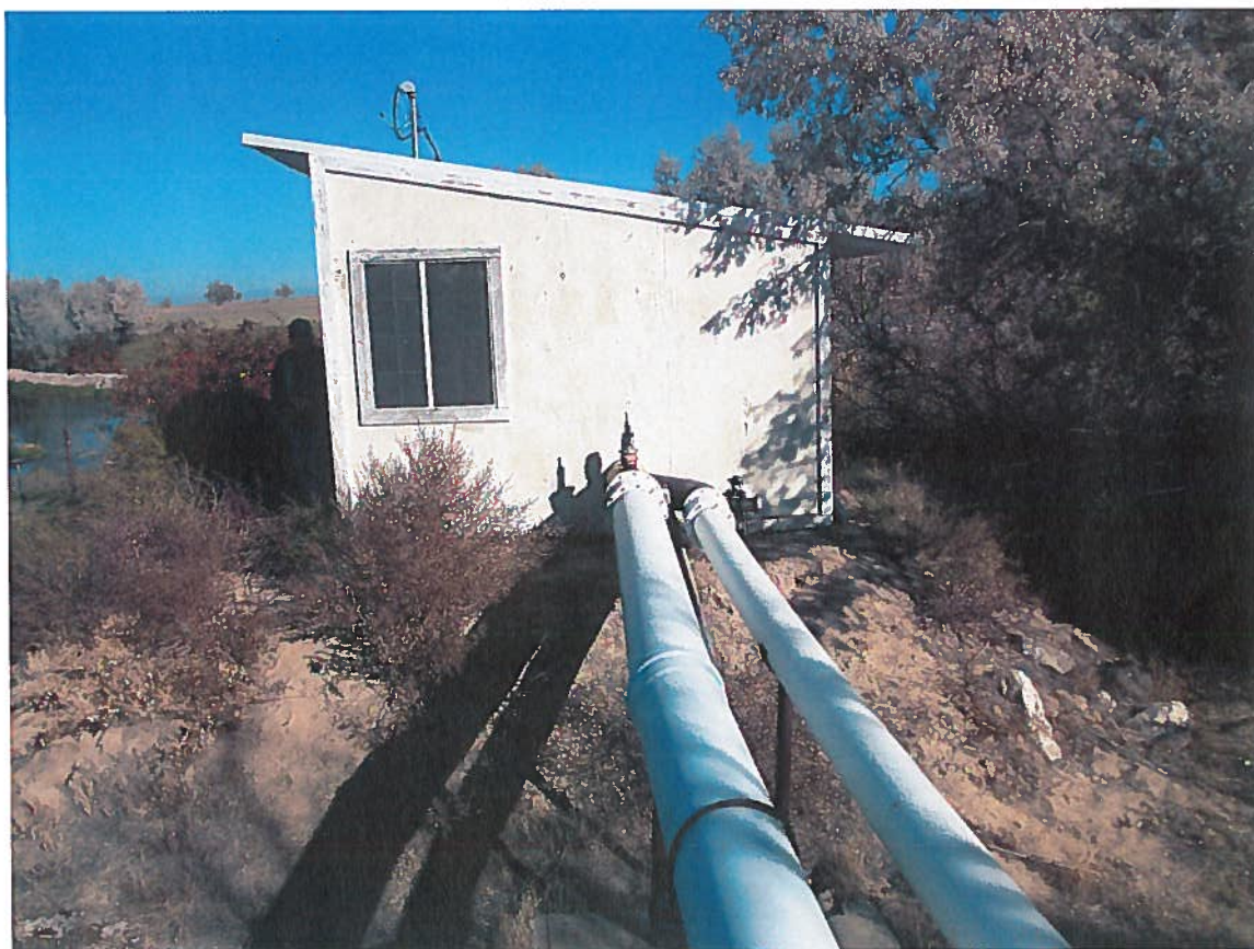
POU - Powerhouse and penstock pipes
