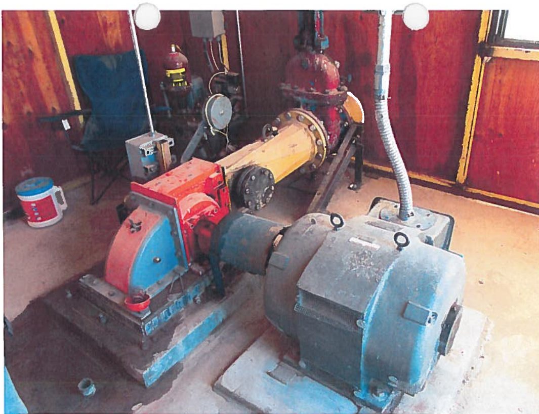
Turbine and generator inside powerhouse
