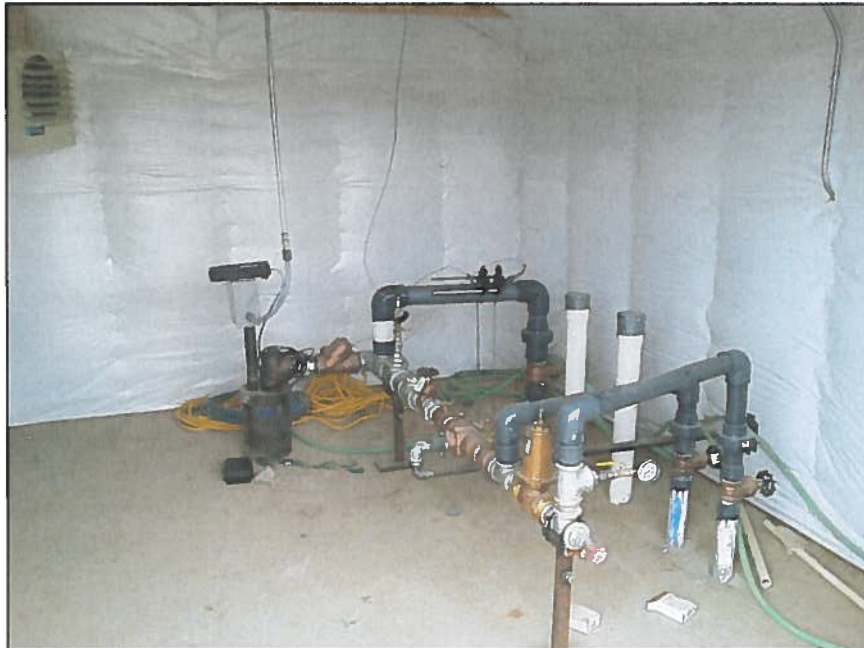
Figure 2: Measured flow was diverted through one mainline to the distribution system.
