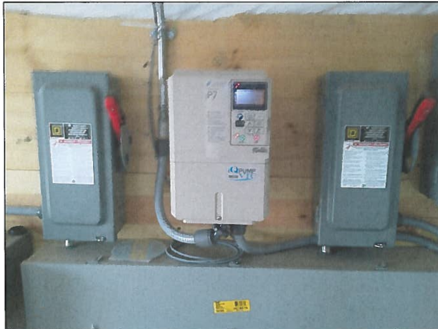
Figure 4: Variable frequency drive controls.
