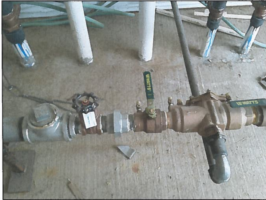
Figure 3: A quarter-turn valve was closed to isolate the measured discharge.
