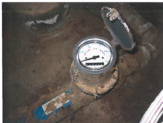
Flowmeter inside dairy barn
