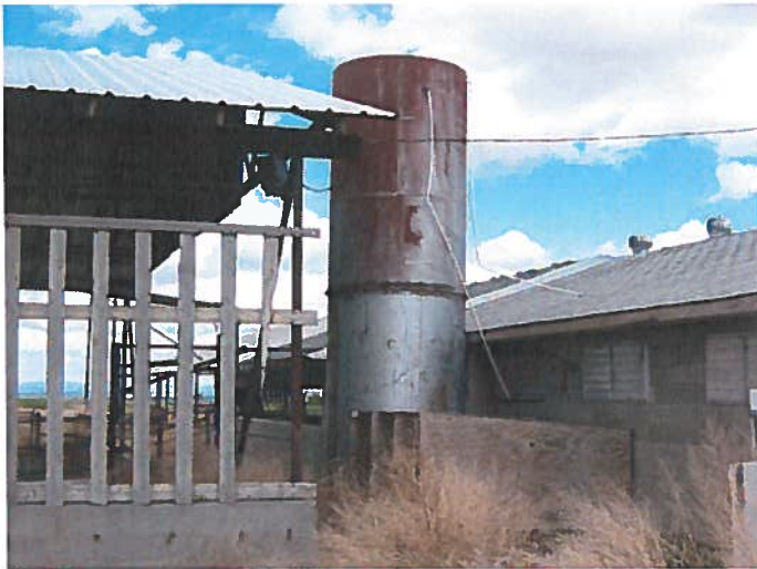
Water storage tank at milking barn
