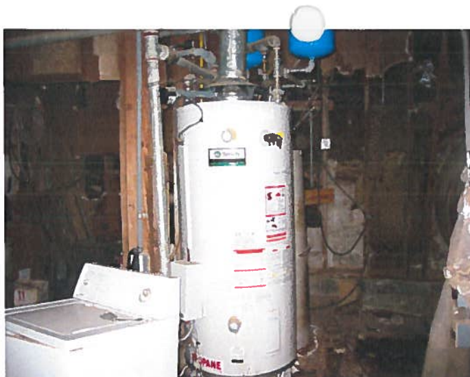
Plumbing inside dairy barn
