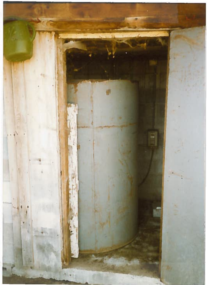
500 gal stor. tank
