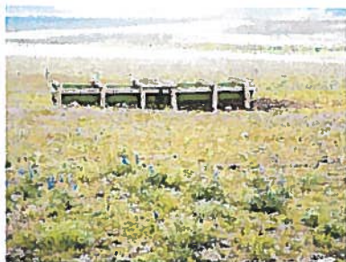
Existing Trough – Weeds Detail
