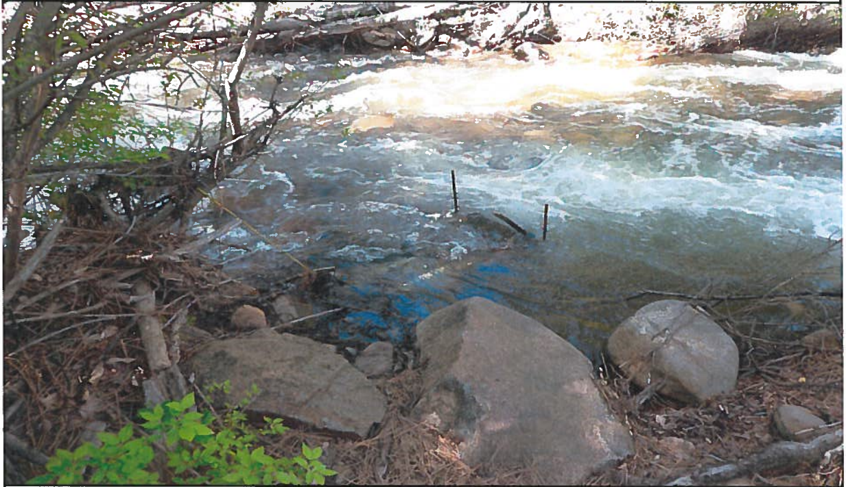
Point of Diversion: View westerly of a screened section of 16" PVC inlet pipe diverting water from Rush Creek to discharge to an open channel.
