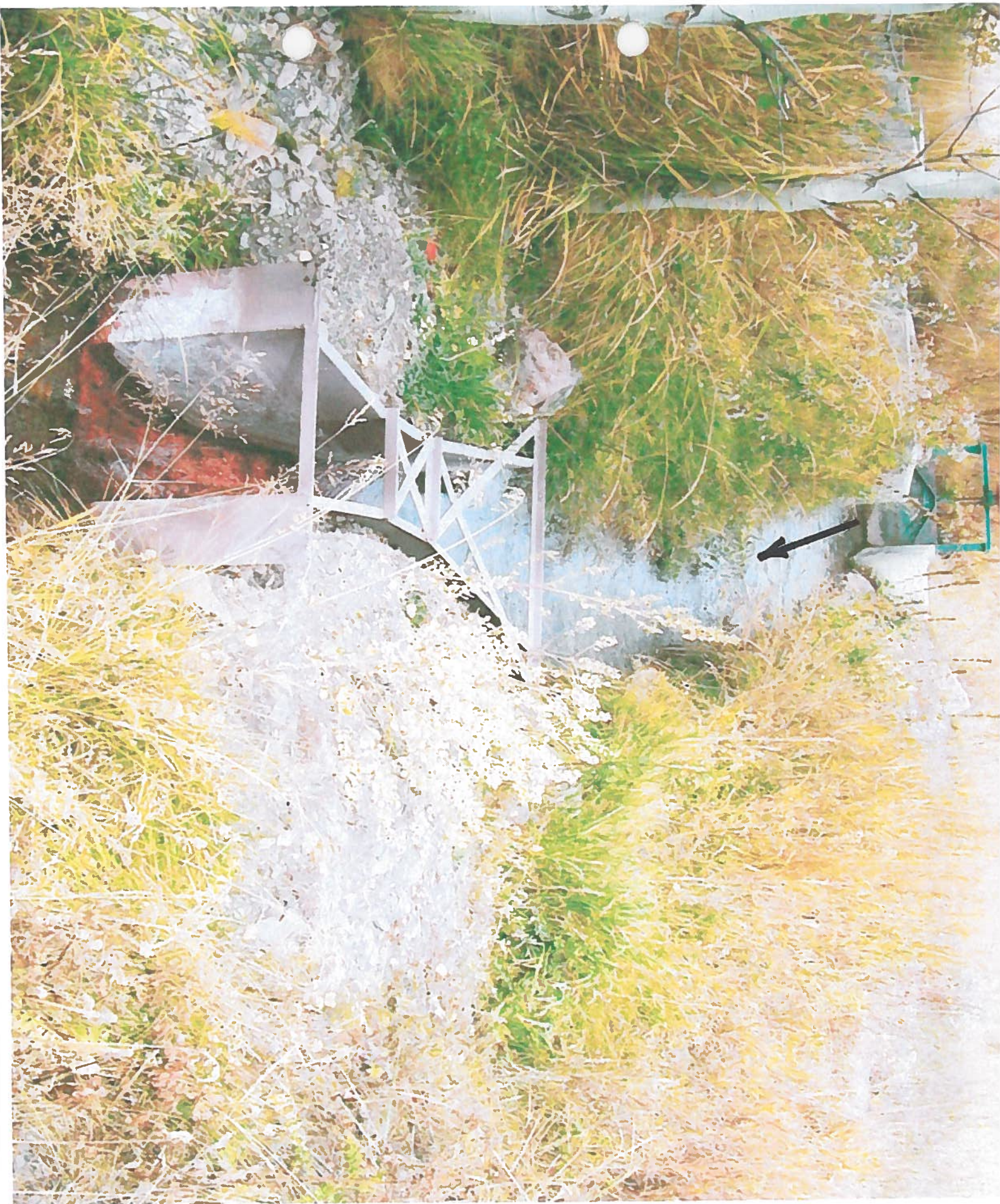
Figure 1 Eagle Creek High Ditch Parshall Flume
