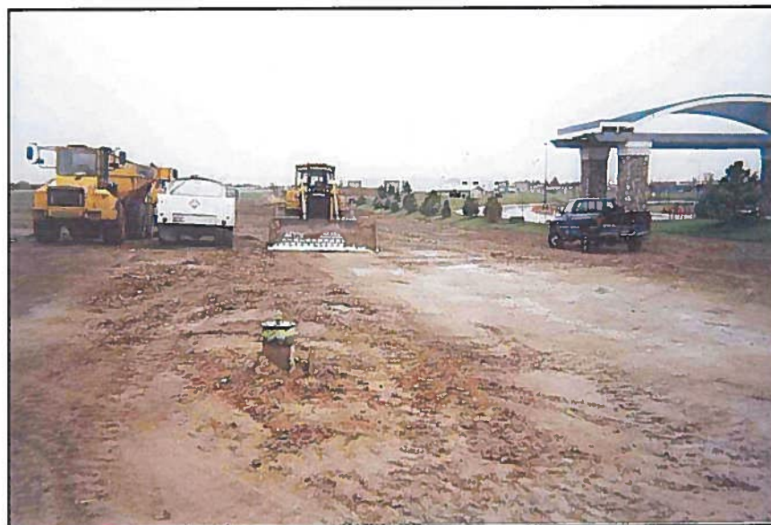
Photograph of the Turfco Well wellhead located 500 feet north of the Meridian Supply Well #23. The photograph was taken March, 2003.
