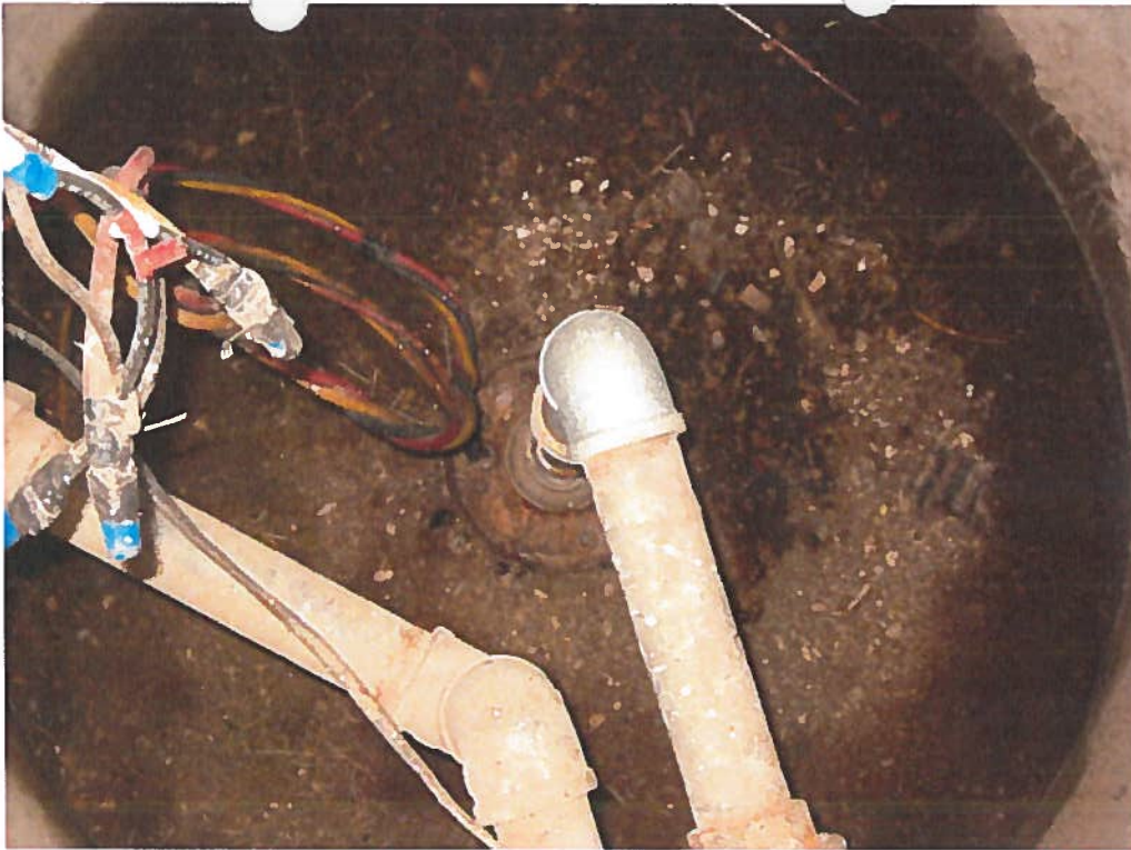
Wellhead and Plumbing inside Well Pit
