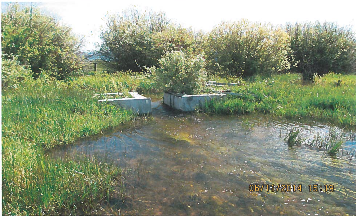
Head-gate off of Dick Creek
