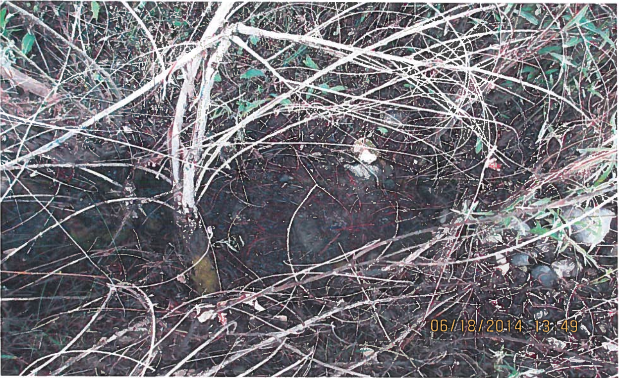
Beginning of Seepage from Chipps Creek Reservoir (-113.939892, 45.172995)
