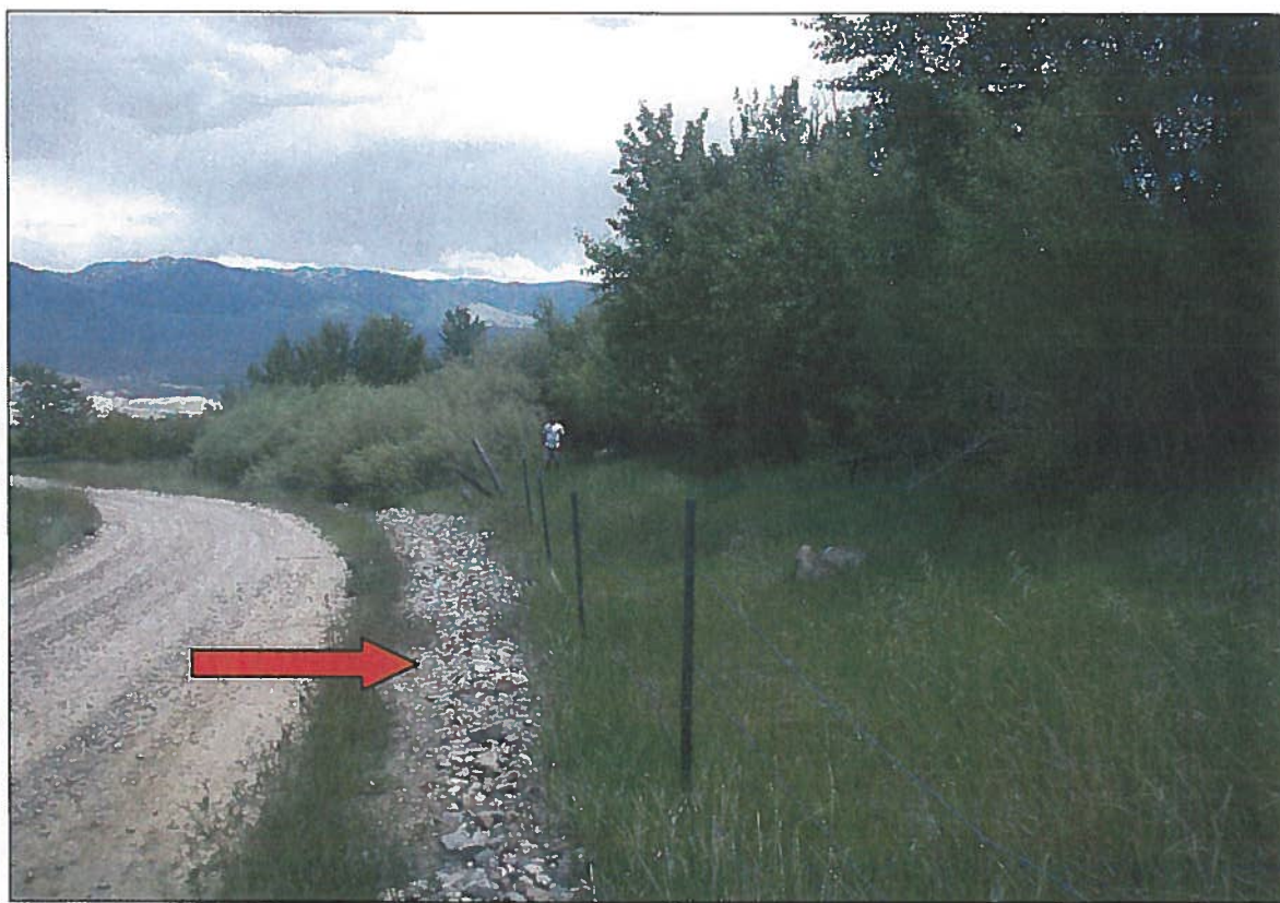
Photo 3 (6/25/09) - Oliver Road, looking east along the north side of the existing embankment. Seepage from the toe of the slope is collected in the gravel drain material (shown by arrow). Note the heavy growth of trees and brush on the downstream slope of the dam.
