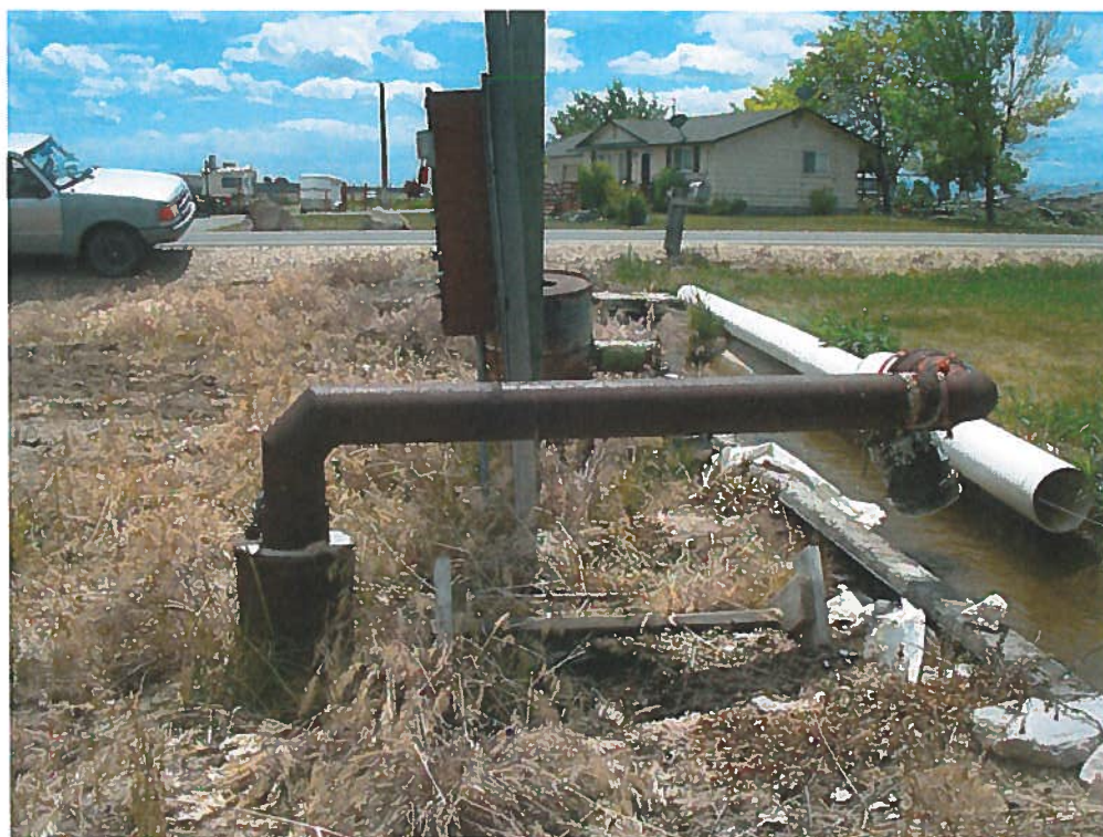
63-11707 Exam 5/23/2012: POD well with discharge piping into cement ditch facing south, Kuna Rd in photo background.
