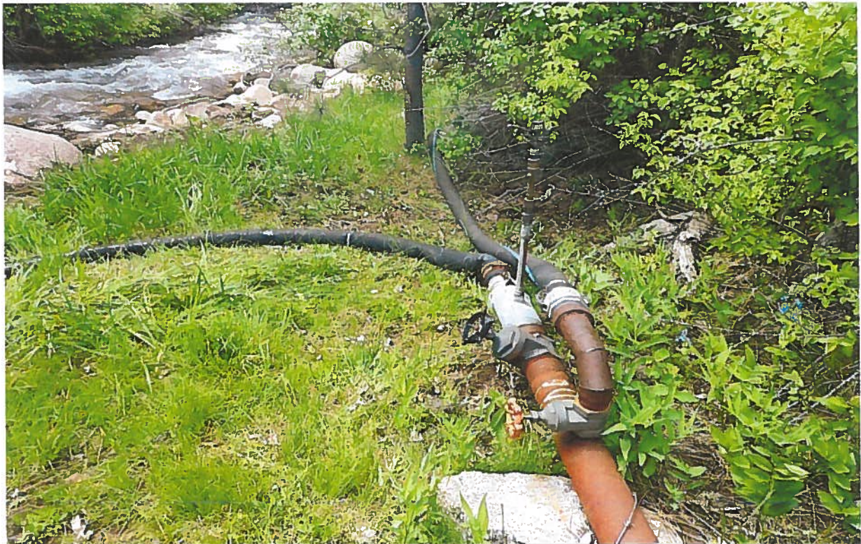
View southwesterly of the 4" supply lines. The 4" flexible hose adjacent to East Pine Creek conveys water to the sprinkler system adjacent to the home site. The 4" steel supply line conveys water to the 3" hand lines in the pasture areas.
