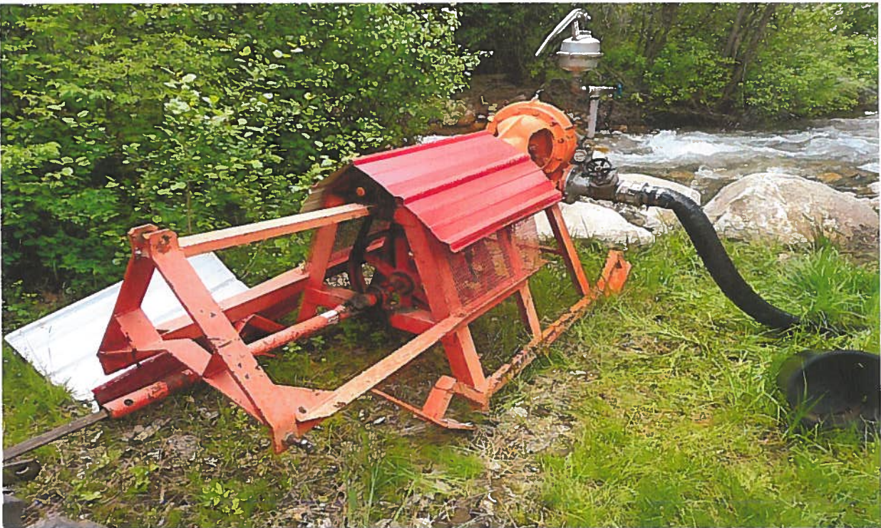
View southwesterly of the pump and mechanical equipment to operate the pump. A 30 or 35-hp Great Bend tractor operates the drive shaft to the mechanical equipment.
