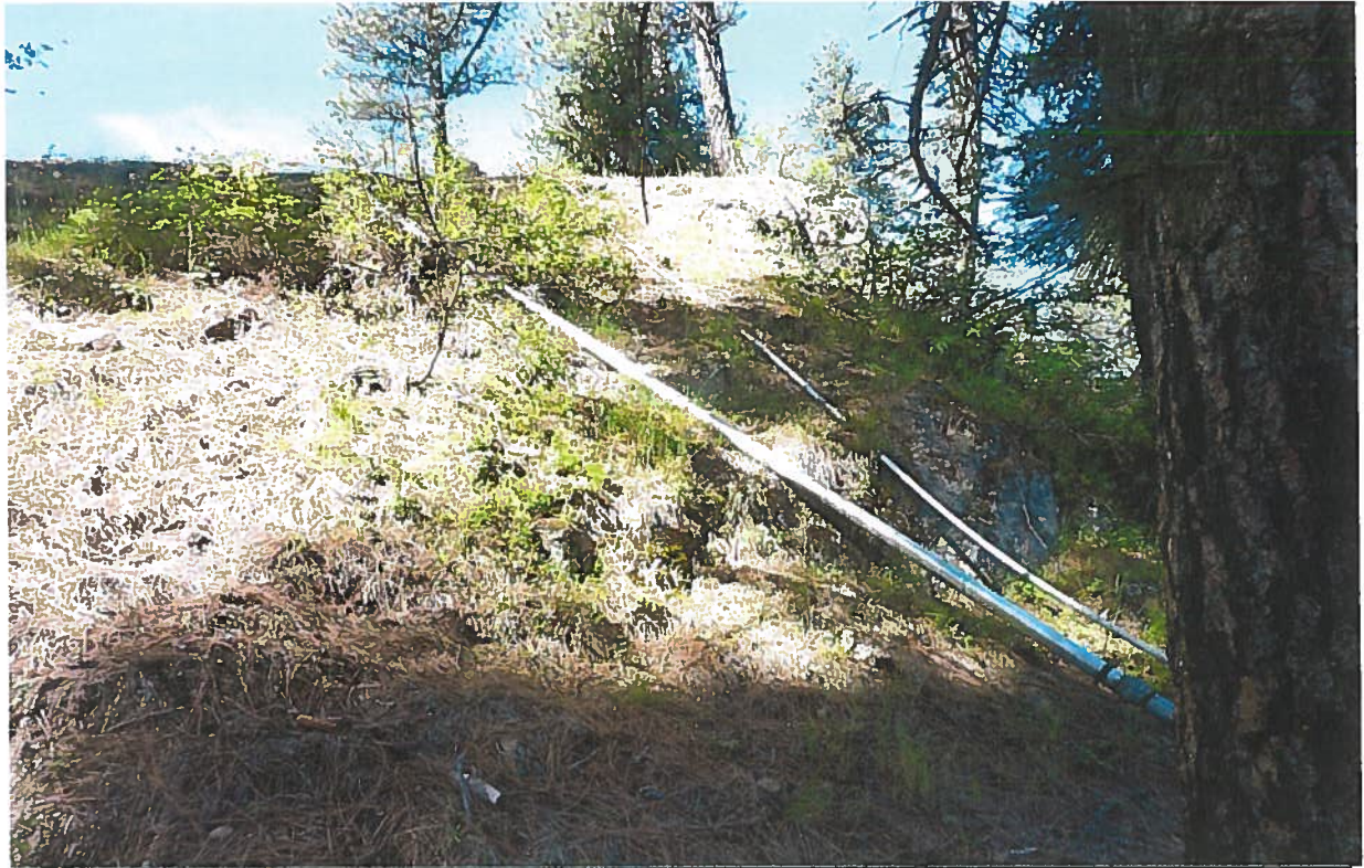
View westerly of the 3" steel main line extending up the river bank to the right holders property above the river.
