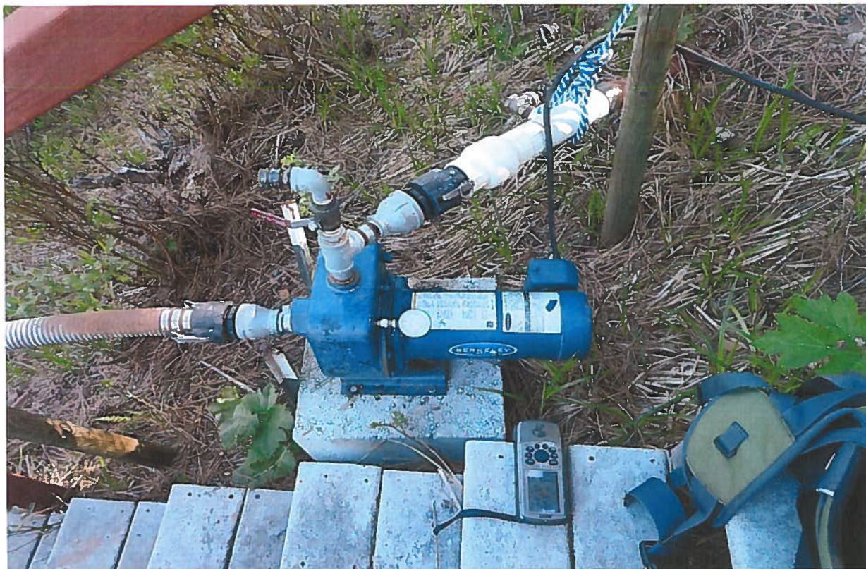
View northerly of the Berkeley centrifugal pump next to the steps. Water is discharged through 2" PVC main line to the 2" handlines. The river pump provides supplemental irrigation water when the Lightning Creek water system is not in operation.
