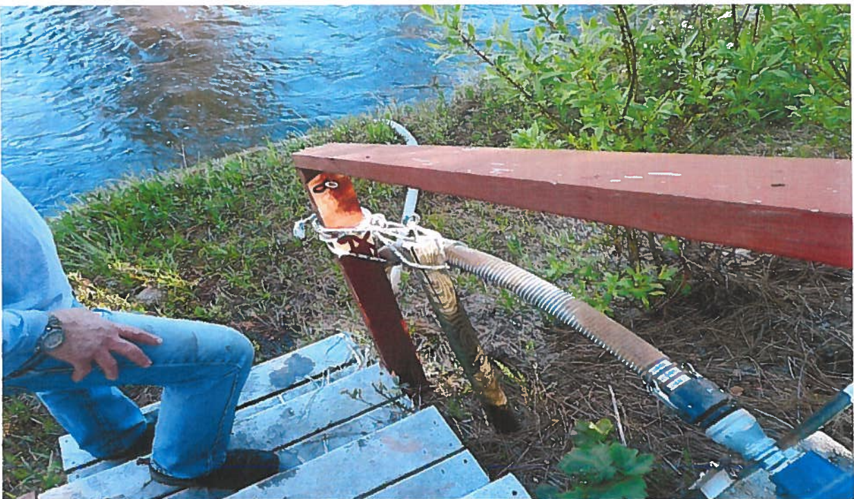
View westerly of the 2 ½" flexible suction line from the river to the Berkeley centrifugal pump on the river bank.
