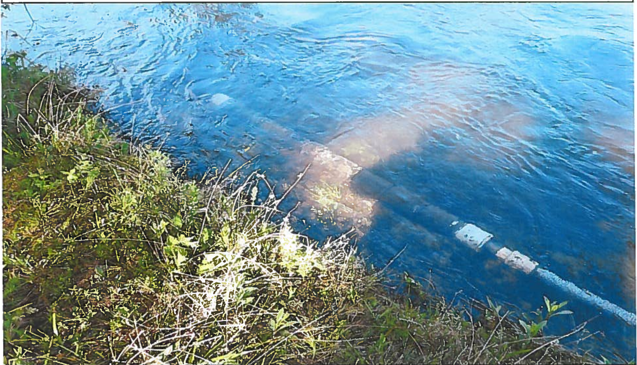
Point of Diversion: View southwesterly of the 4" PVC perforated intake pipe and the 2 ½" flexible suction line near the east bank of the Middle Fork of the Payette River.
