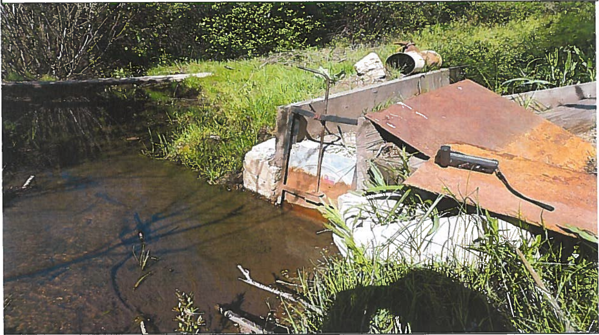
Point of Diversion: View westerly of the concrete diversion structure and 12" slide gate. Water is conveyed through a 4' section of 12" concrete pipe to a concrete channel containing a Cipolletti weir for flow measurement.
