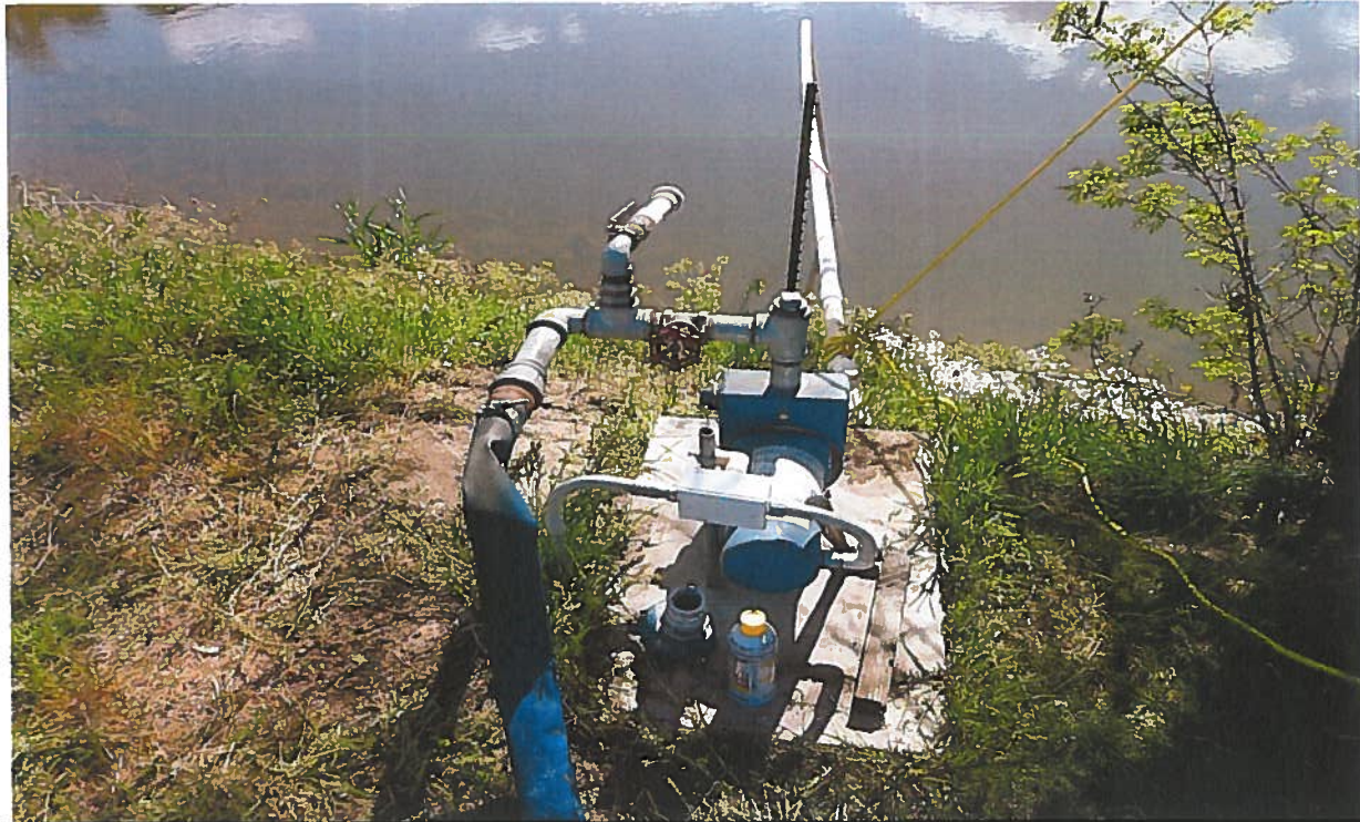
View easterly of the 1-HP centrifugal pump and 1 1/2" PVC suction line. Water is conveyed through a 2" flexible hose for flood irrigation of pasture land.
