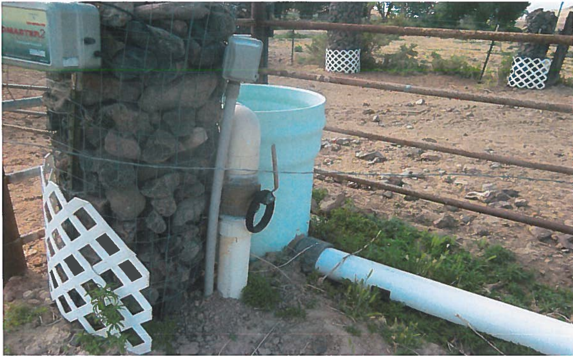
Riser at southeast end of field. Also seen is the 6 " gated pipe.
