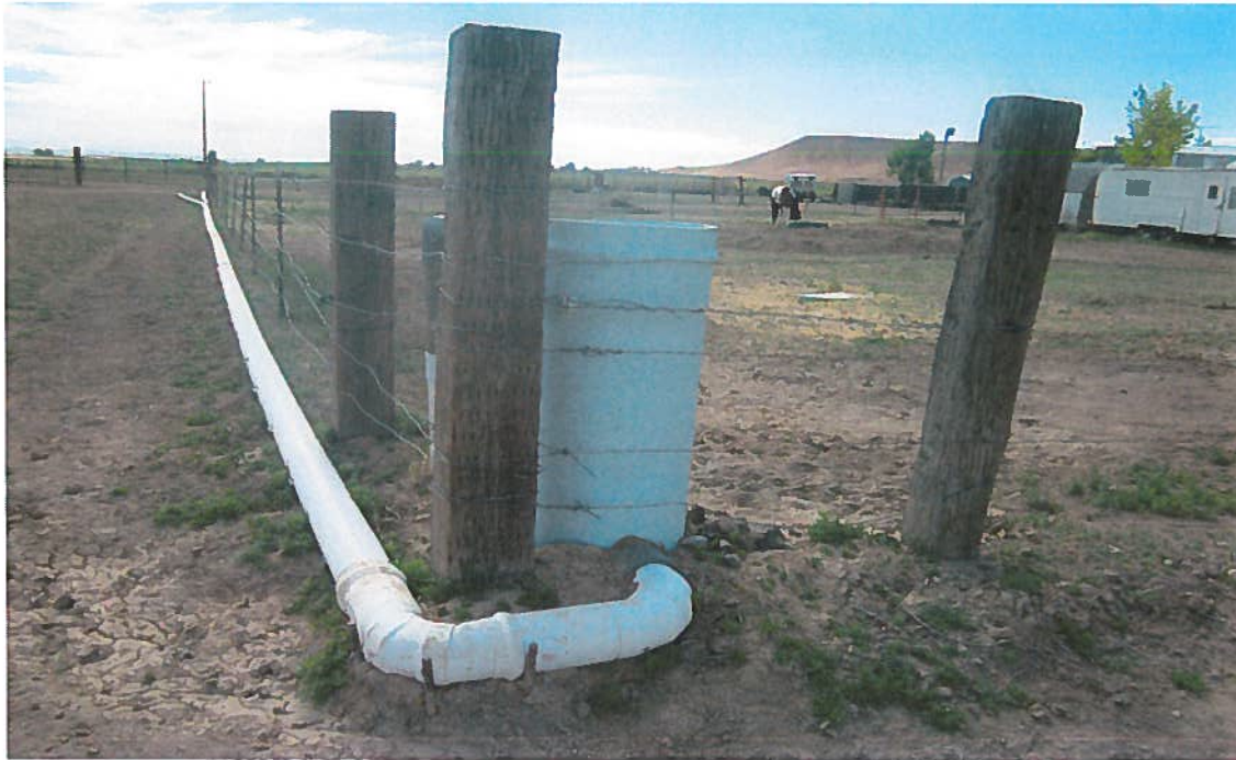
Looking at the riser north of the well, and the 6 " gated pipe that irrigates the northeast field.
