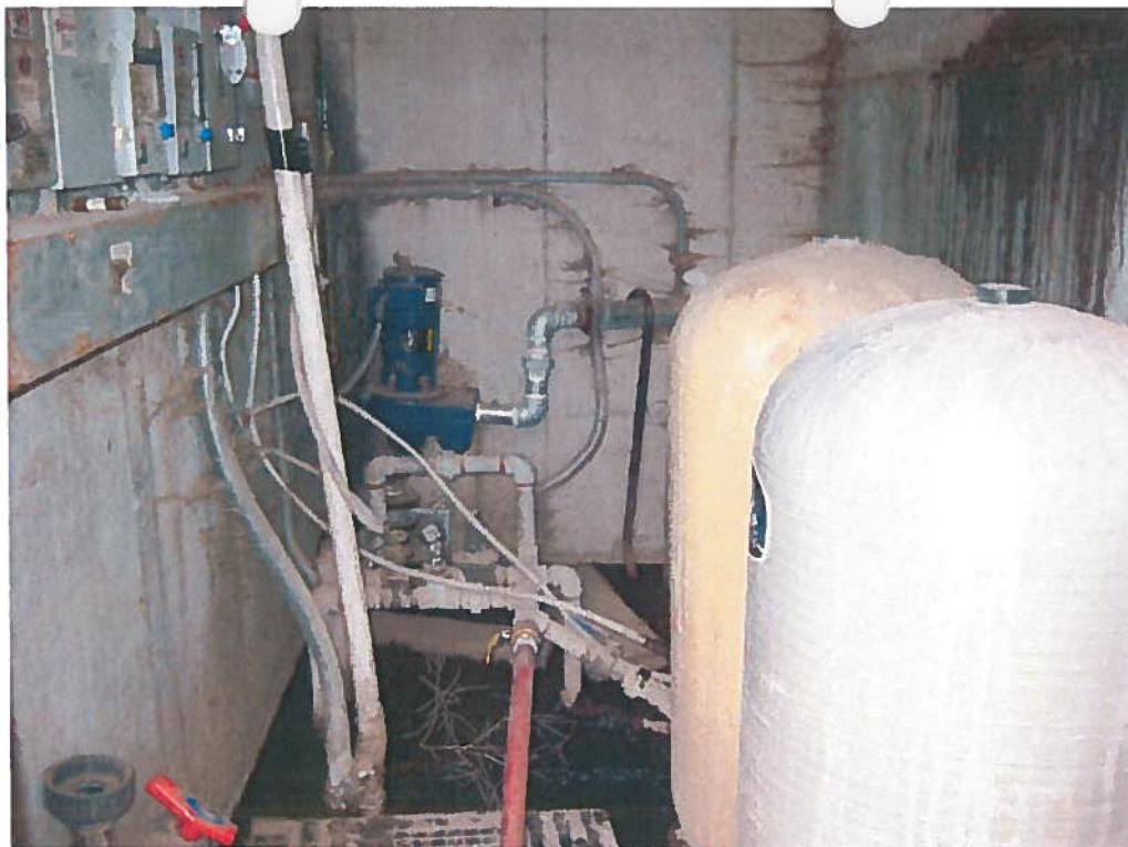
Plumbing inside Pump House
