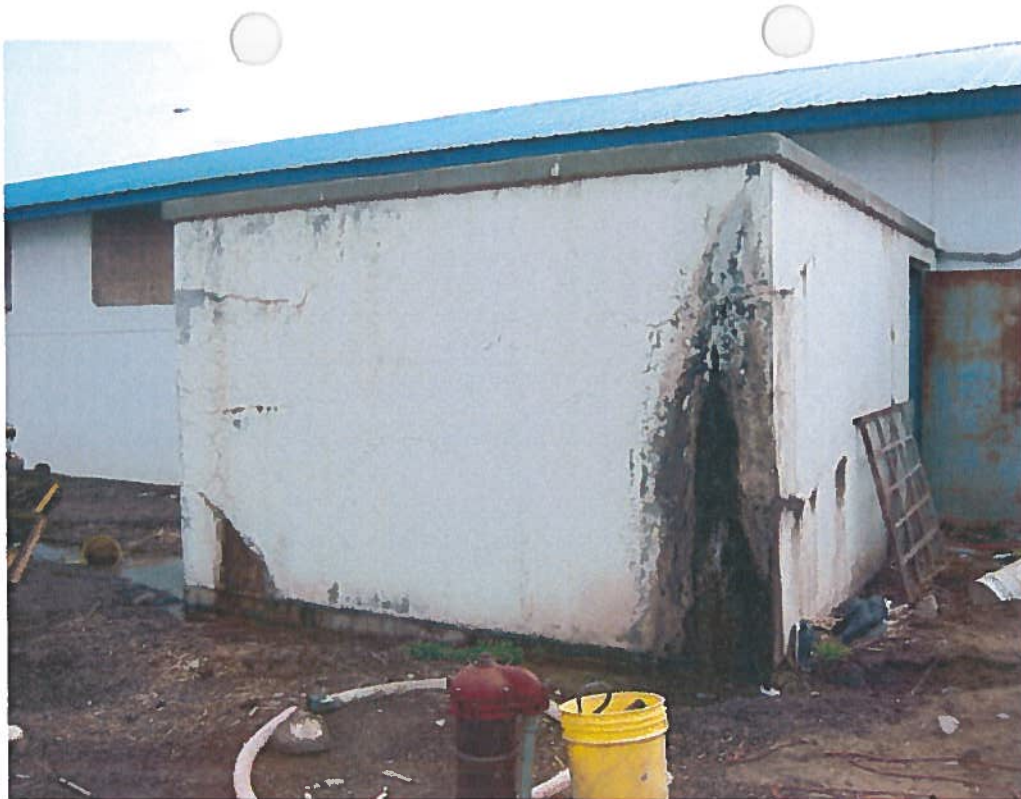
Water Storage Tank and Pump House (Behind)
