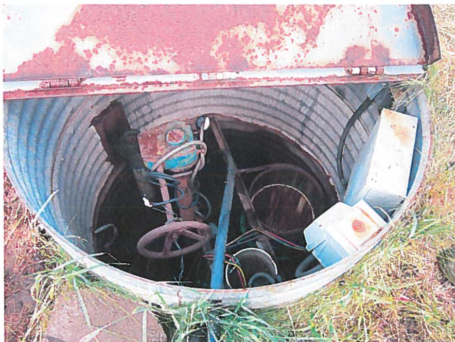
Figure 2: Recirculation system in culvert.
