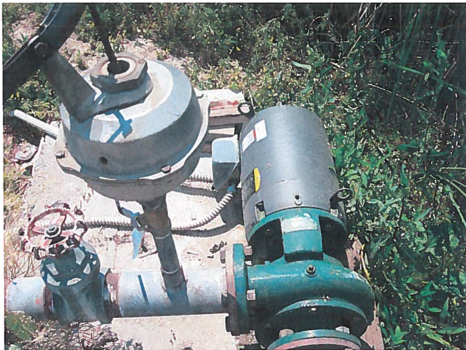
Figure 1: 15 Hp pump adjacent to the pond.
