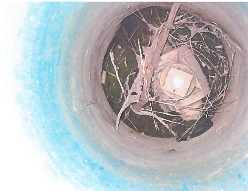
Control valve inside box.
