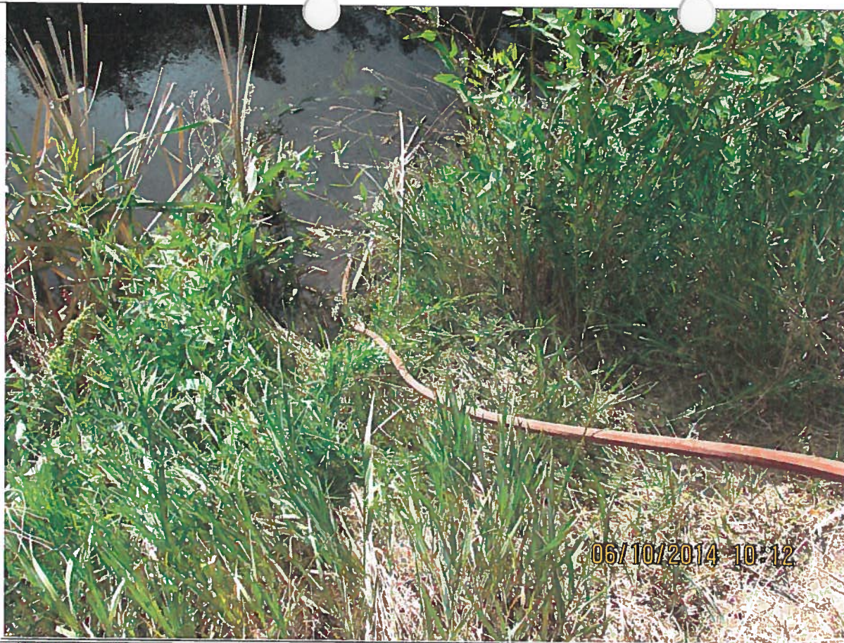
Hose with a cage rests inside the creek.
