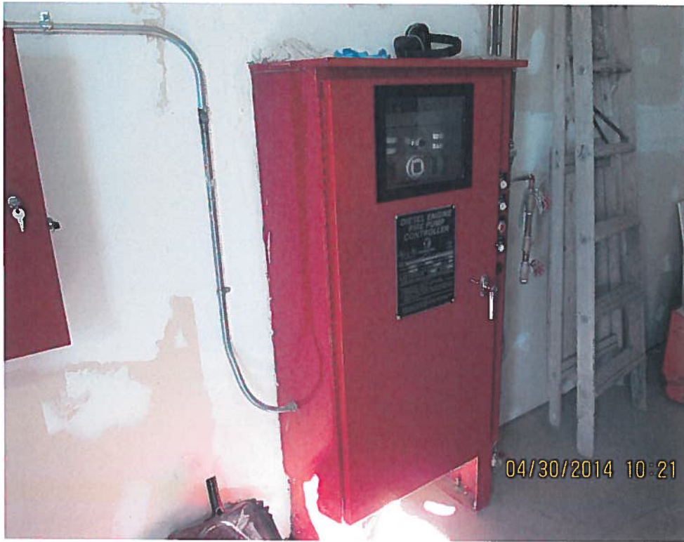
Motor control panel in storage house.
