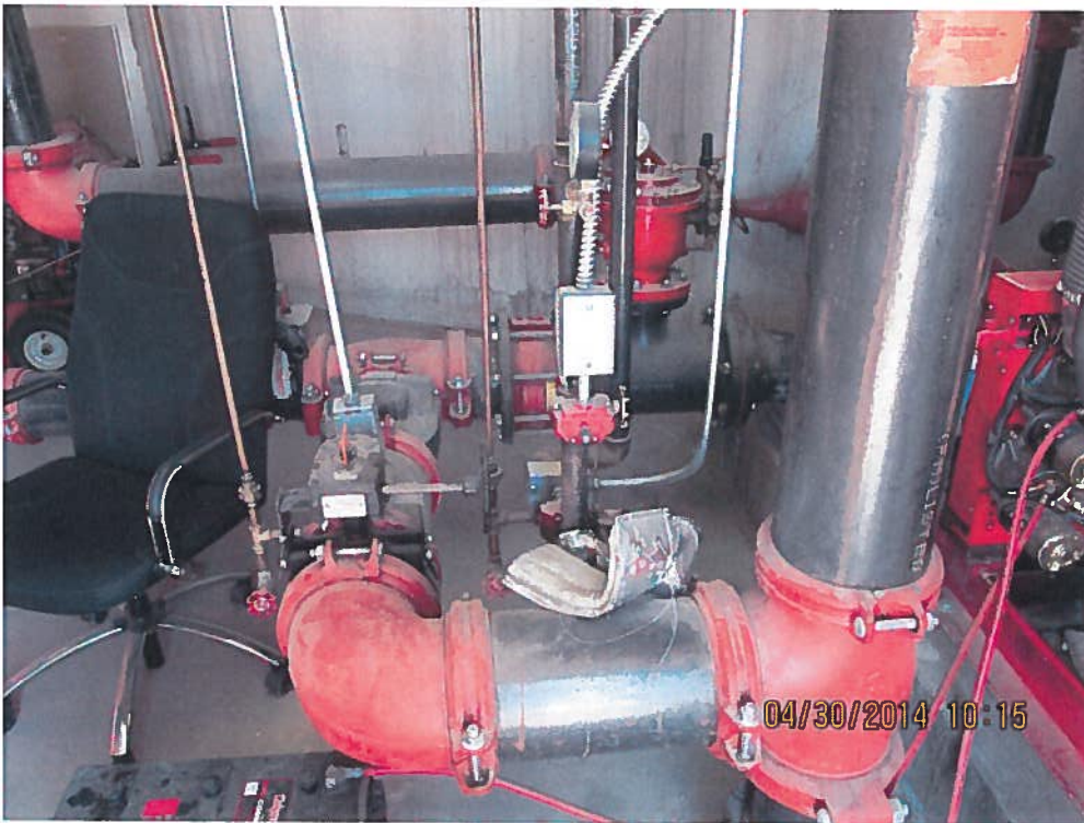
Storage pipes are closed circuit which allows user to test system without losing water. Water circulates back into tank.
