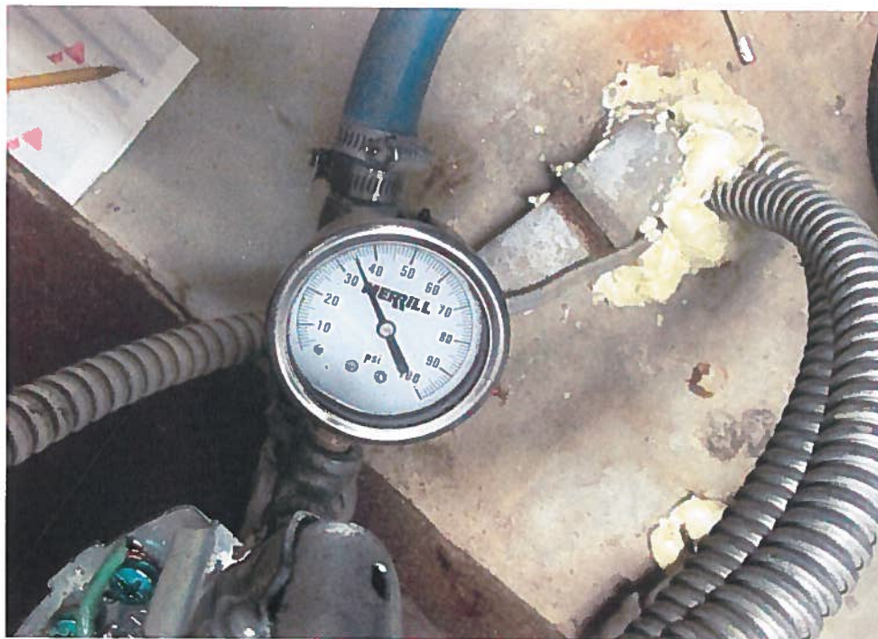
Gauge in storage house reads 35 psi.
