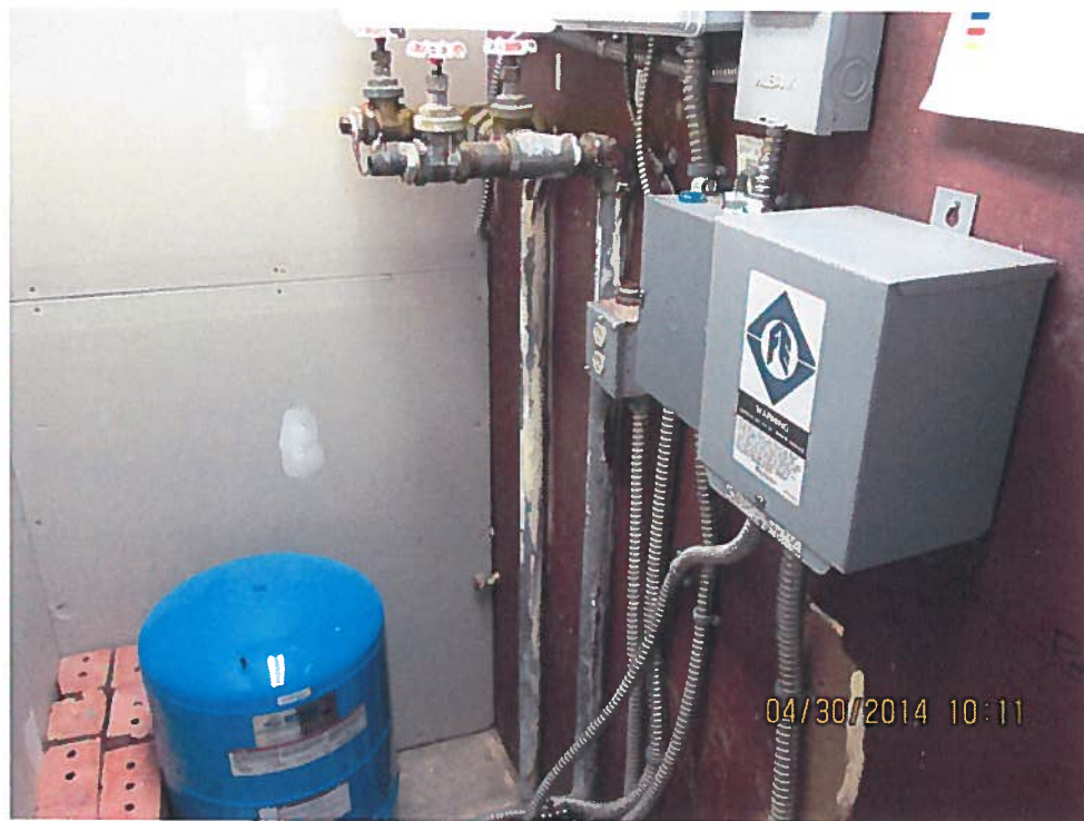
Pump room. Manual switch to storage.
