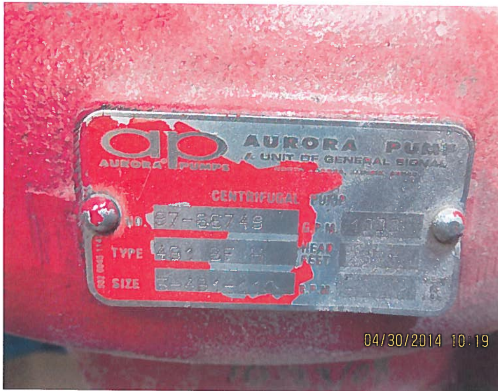
Pump tag in storage house.
