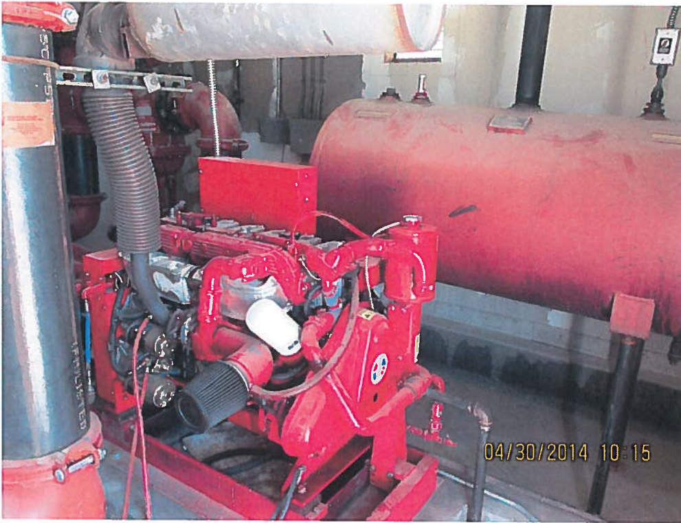
120 hp motor at storage supplies sprinklers with water from storage tank.
