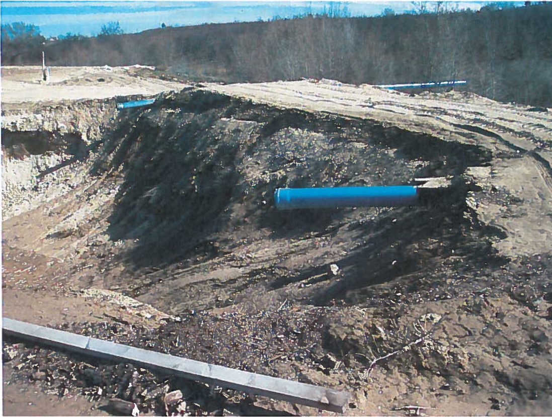
Photo No. 1, viewing upstream slope of dam showing overstep slopes where surface slumping is occurring.
