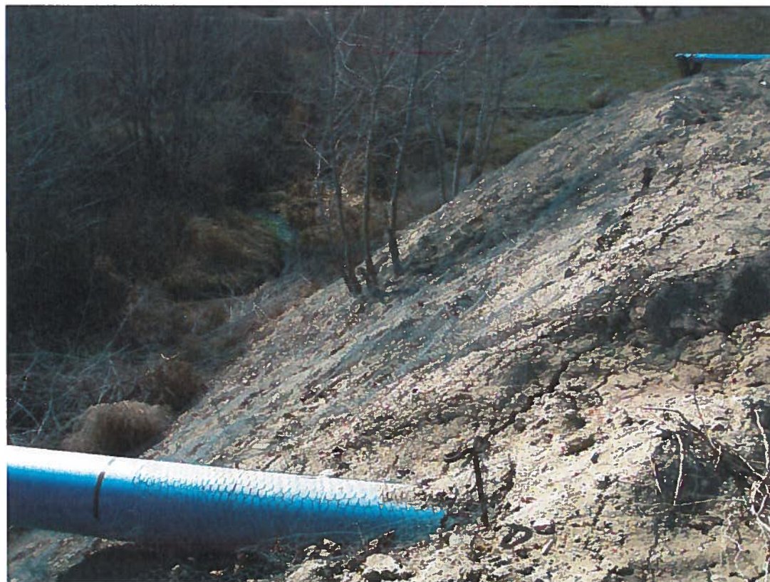
Photo No. 4 viewing downstream slope from left outlet pipe showing tension cracking on downstream face of dam.
