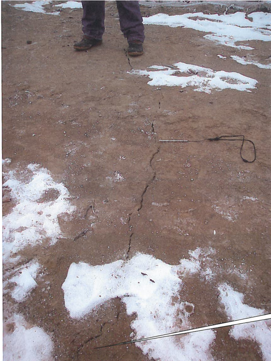
Photo No. 6, developing continuous crack through right abutment contact area indicating differential settlement of embankment soils.
