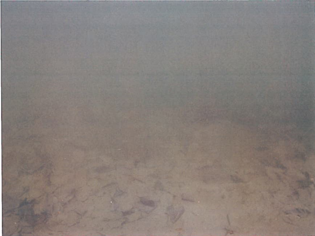
Photo No. 4, close-up of upstream face showing a bench and then a vertical drop-off of the dam's upstream slope.
