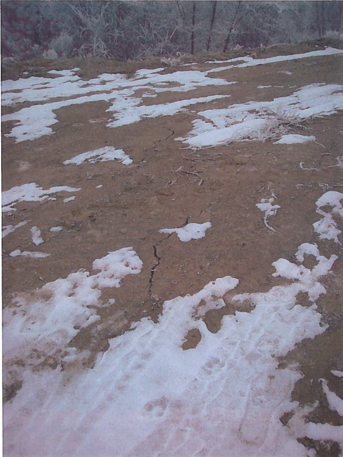
Photo No. 7 viewing downstream at left abutment continuous crack developing on embankment crest.
