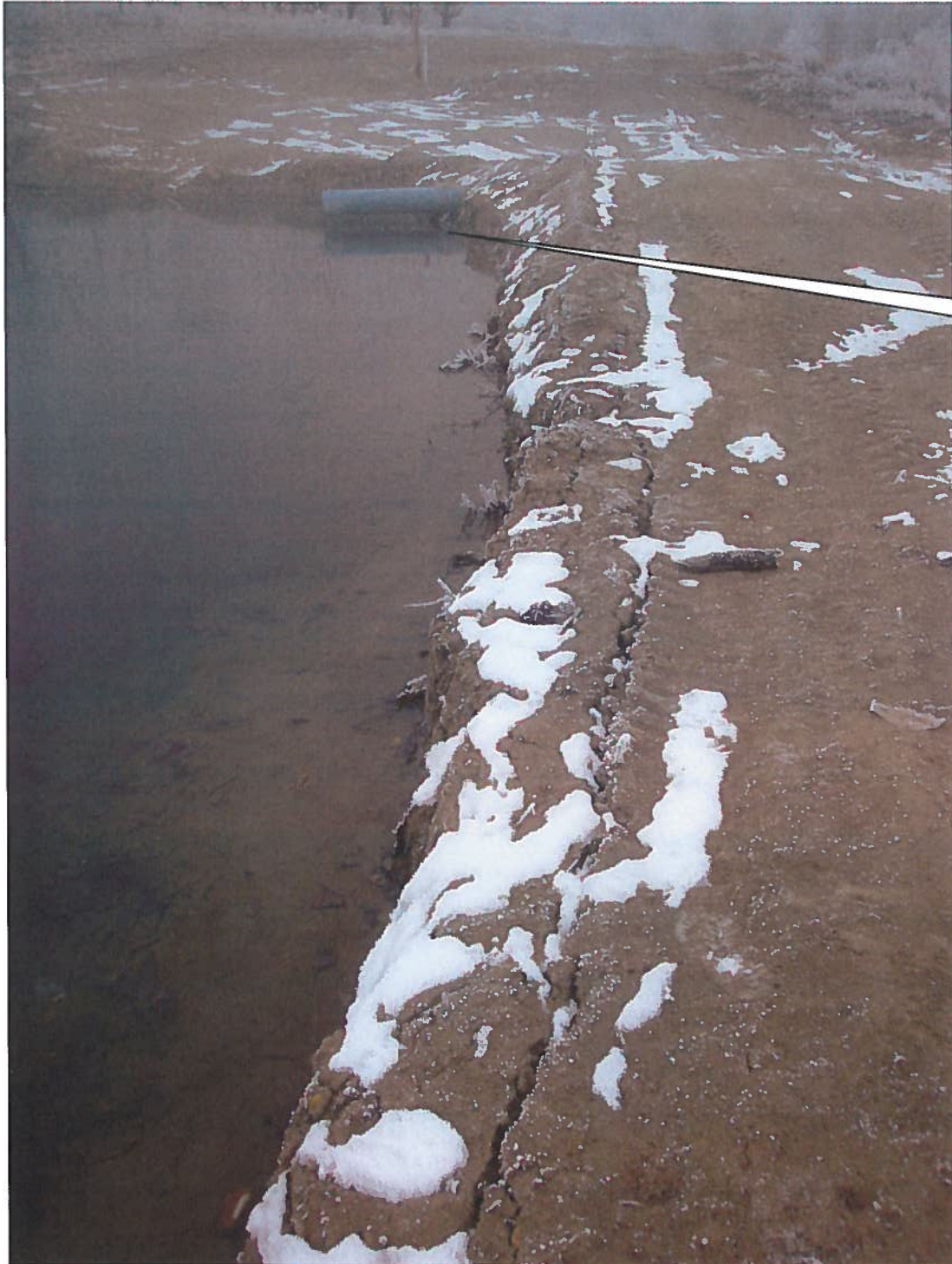
Photo No. 3, viewing upstream face of dam at over steep slope resulting in cracking and slumping of embankment crest
