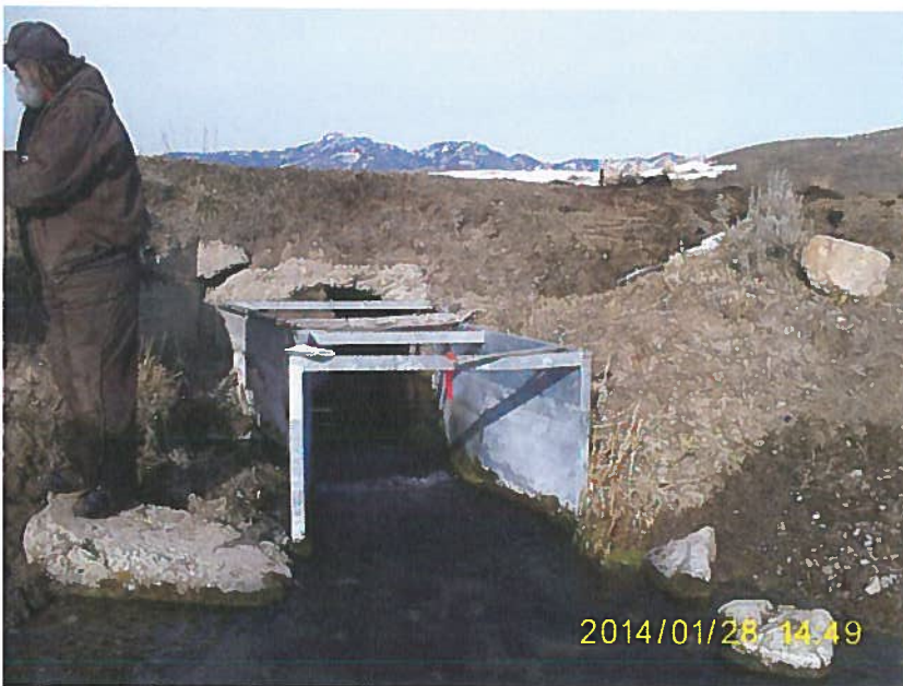
Photo 7769. Three foot Parshall flume on the outlet of Illum Spring.
