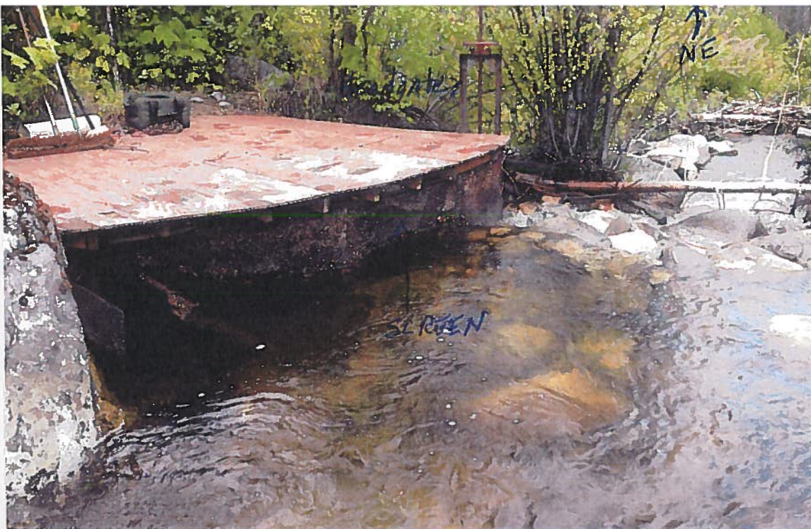
Point of Diversion: View northeasterly of the screened intake structure on Lemhi Creek. The wheel gate controls flow to a collection box for conveyance thru the 8" PVC penstock.
