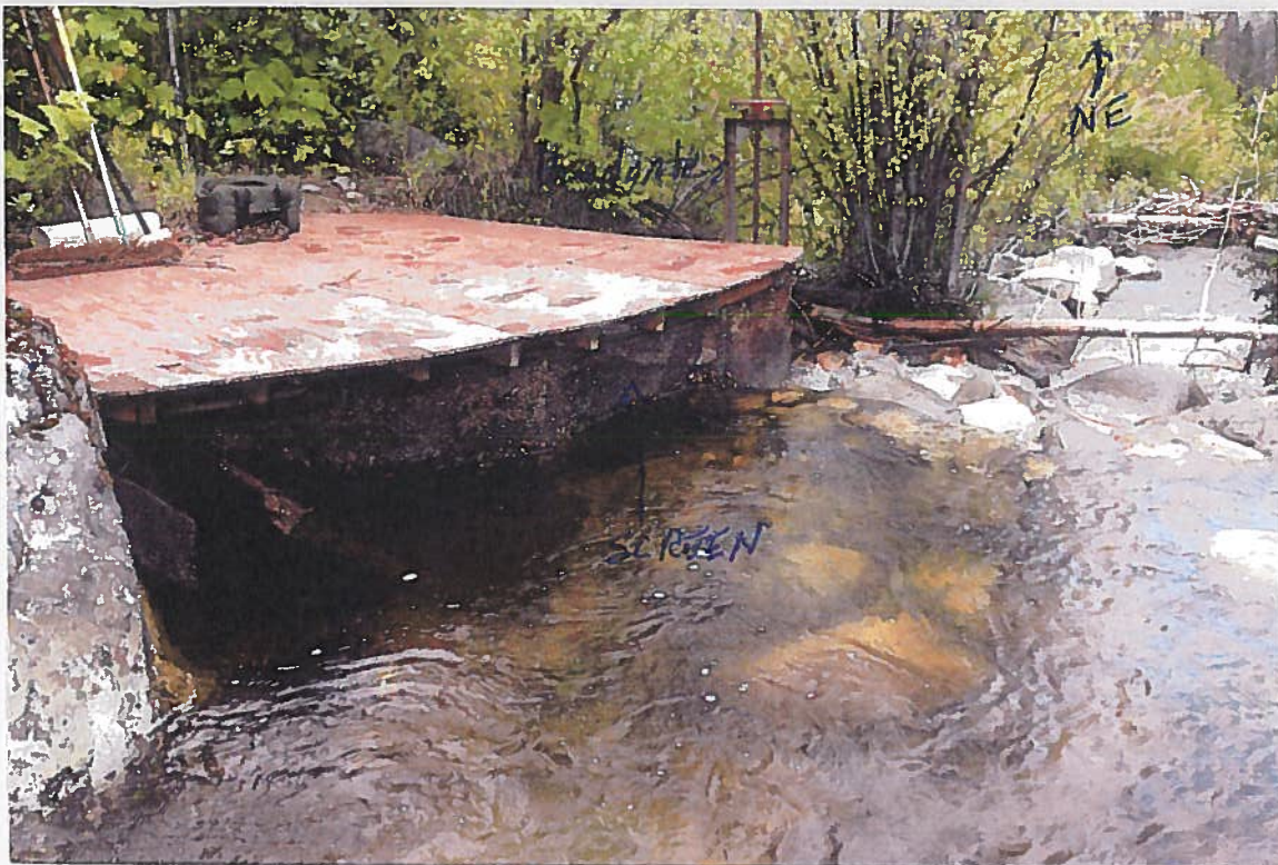
Point of Diversion: View northeasterly of the screened intake structure on Lemhi Creek. The wheel gate controls flow to a collection box for conveyance through the 8" PVC supply line.
