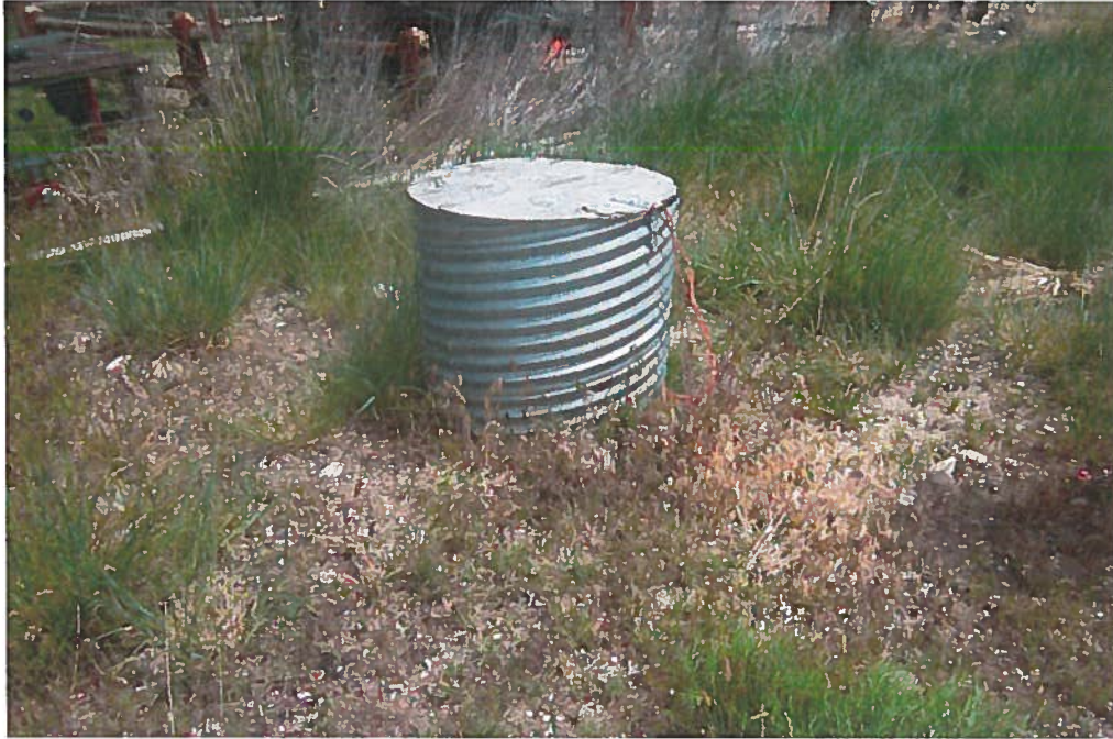
The corrugated metal pipe that encloses the well pipe.
