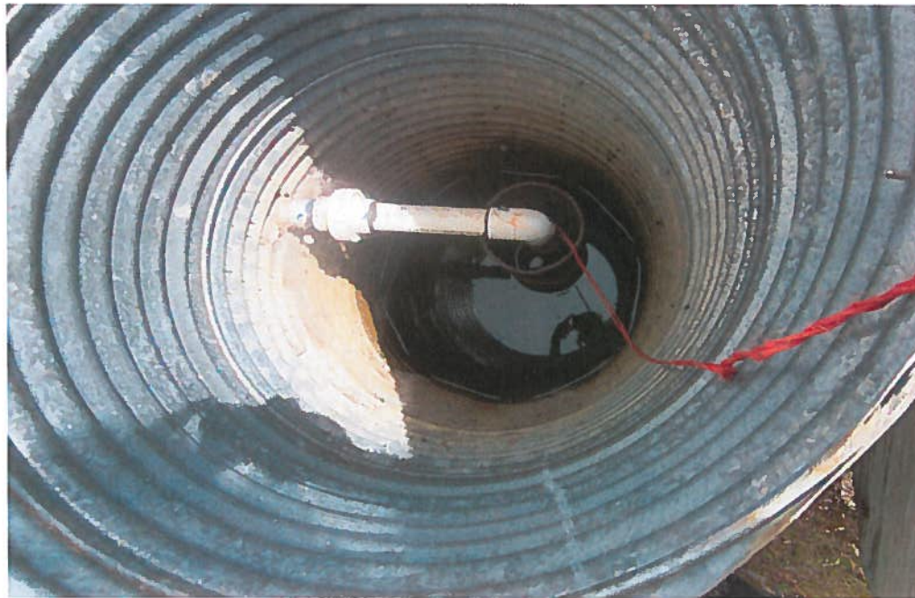
Well pipe and 2" PVC pipe to pump seen.
