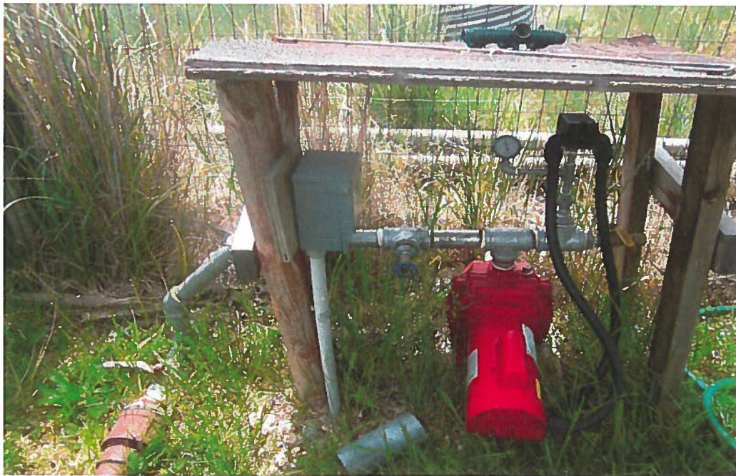
Piping seen left connects to hand line.
