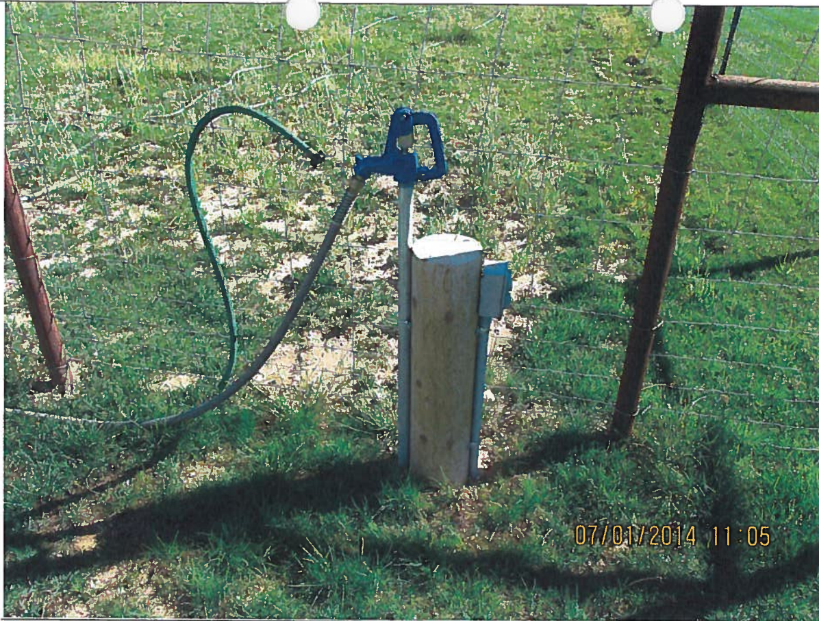
Spigot connected to the system.
