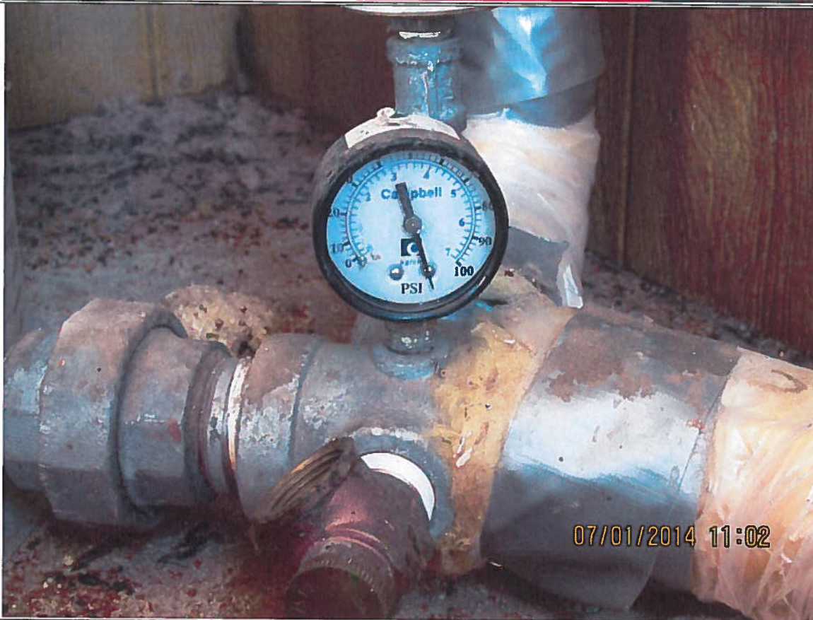
psi gauge reads a high pressure. Assumed to be broken.
