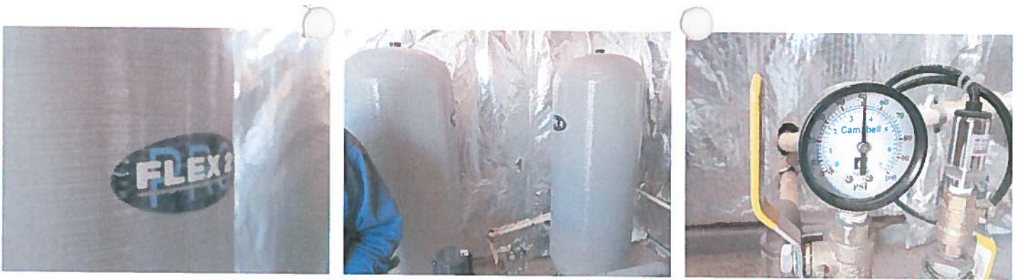
ProFlex 2 pressure tanks are shown (left and center). When pressure reached 50 psi, the pump turned on (right).
