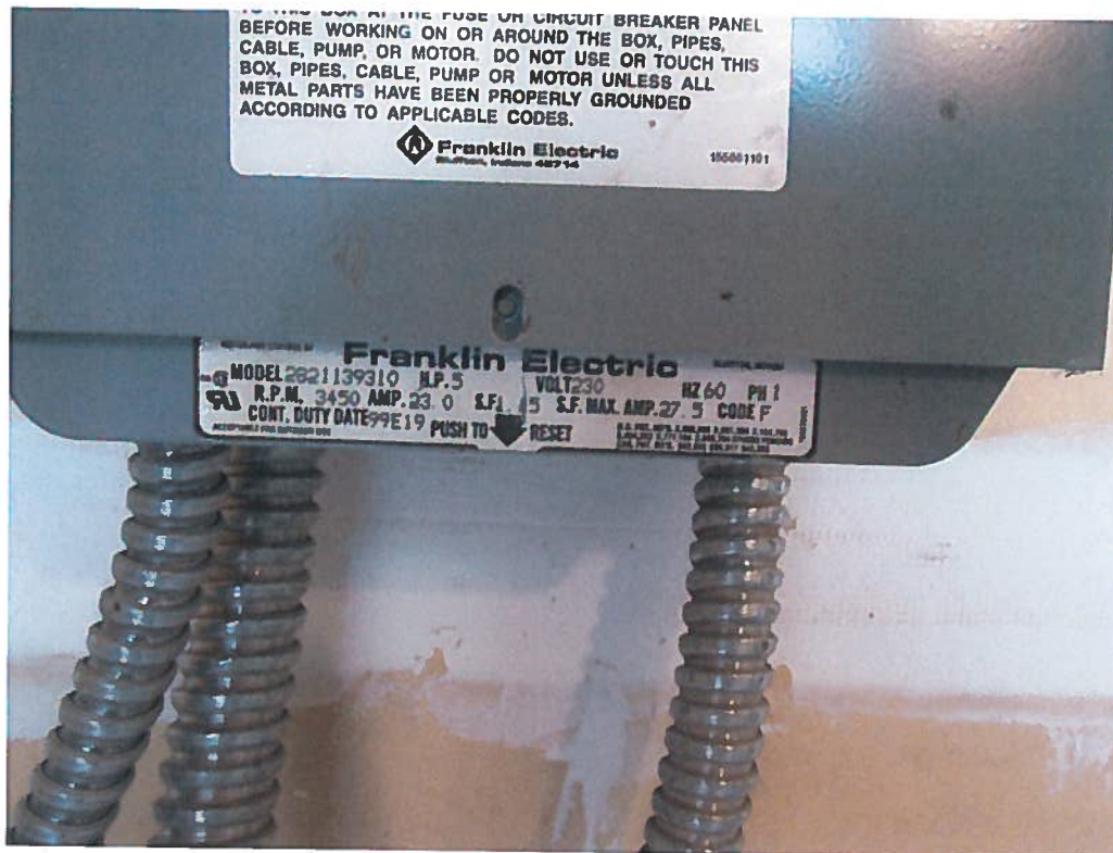
Pump control box
