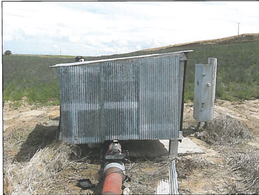
Figure 3: Well #2 facing easterly towards Well #1.
