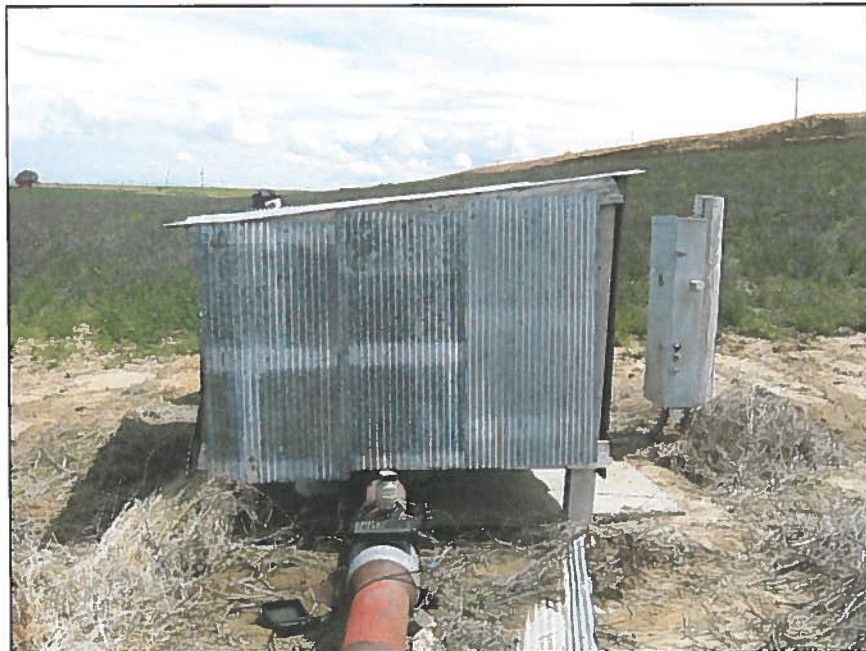
Figure 4: Well #2 facing easterly towards Well #1.
