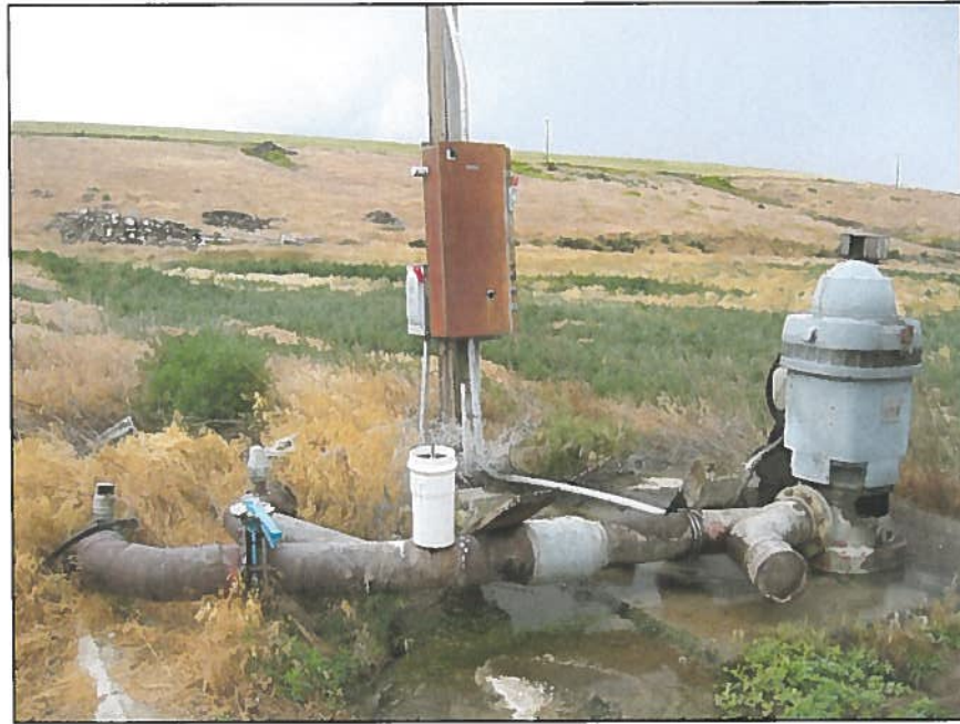
Figure 1: Well #1 facing southerly to a 1/2-pivot on the hill developed under permit 63-33073.
