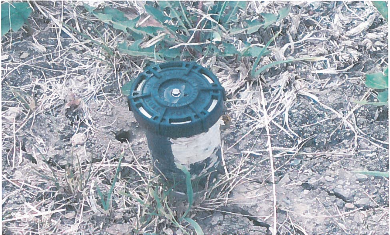
Underground Sprinklers for Lawn South of Home and Parking Area
