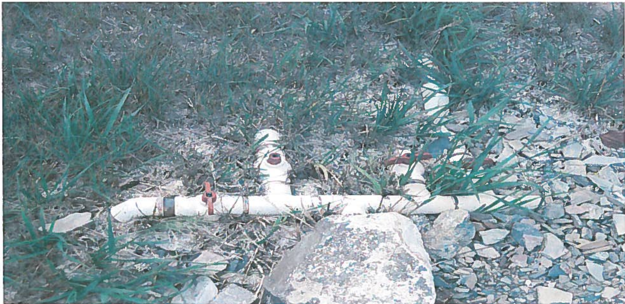
Sprinkler System Valves from Well Head
