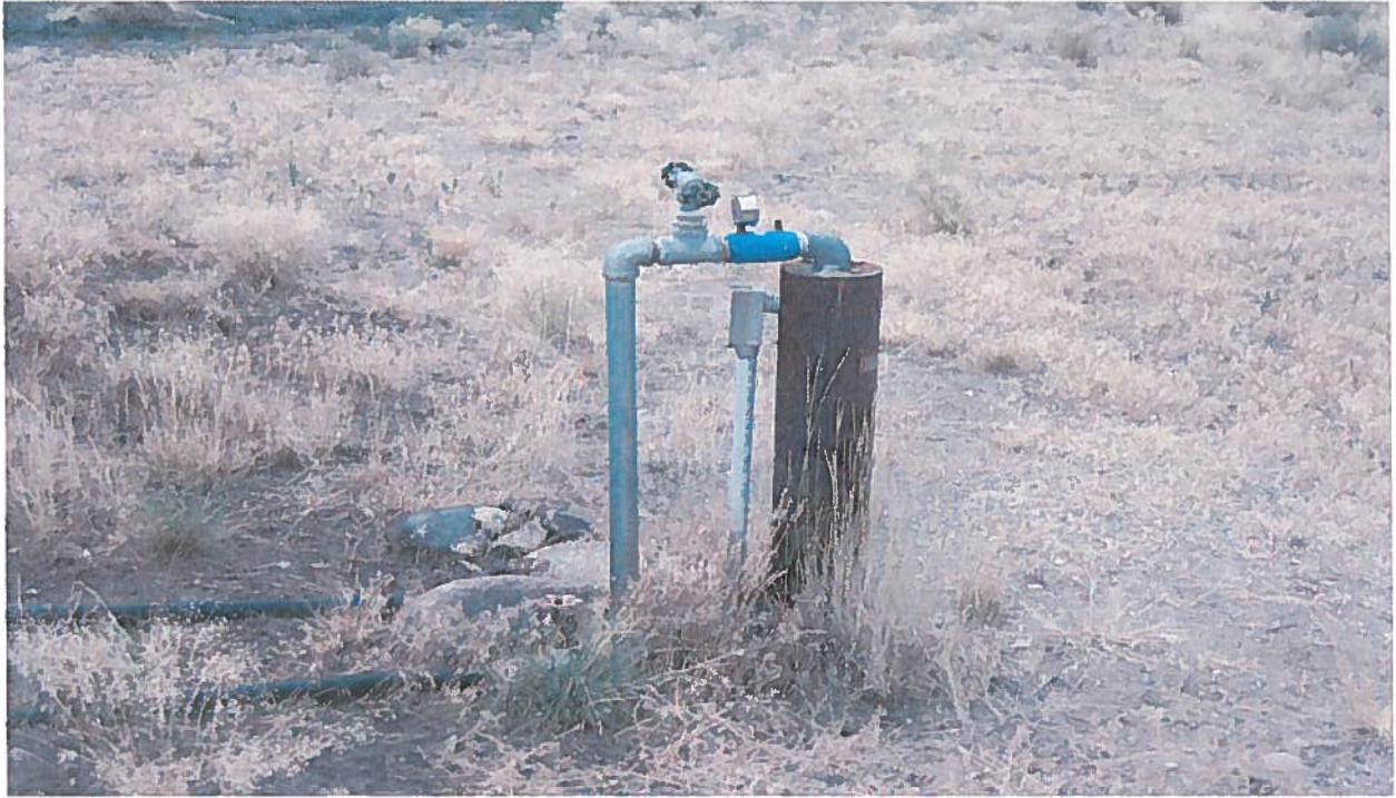
Well Head with 2" Irrigation Lines
