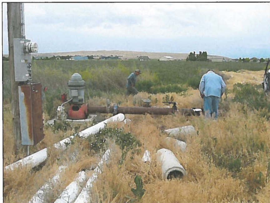
Figure 2: Well facing southerly showing place of use.
