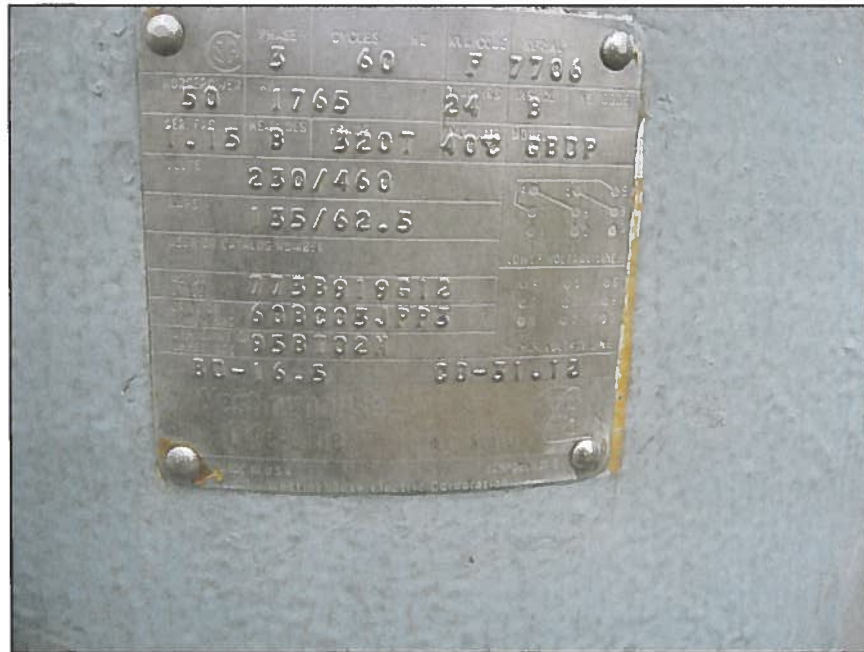
Figure 9: Well #2 motor nameplate.
