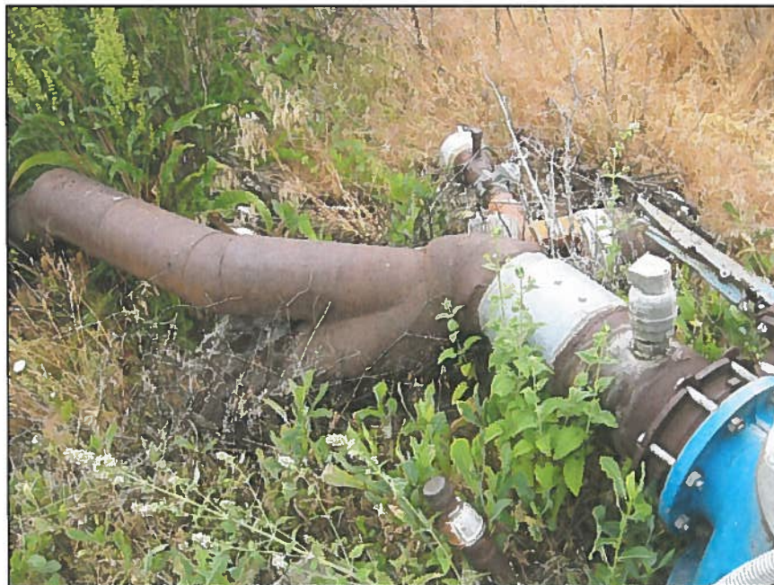
Figure 10: Well #2 discharge plumbing.
