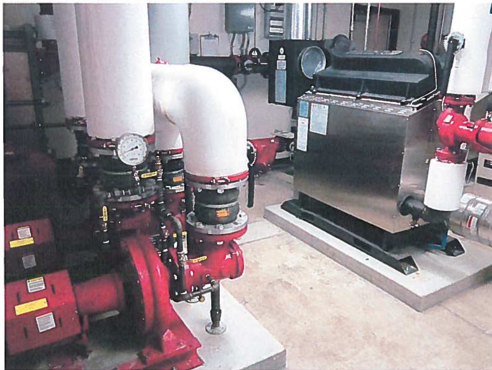
Figure 5: Variable Frequency Drives and Part of Heat Exchange System
