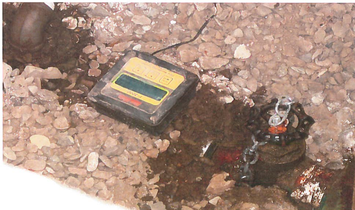
Below: Meter and lockable valve
