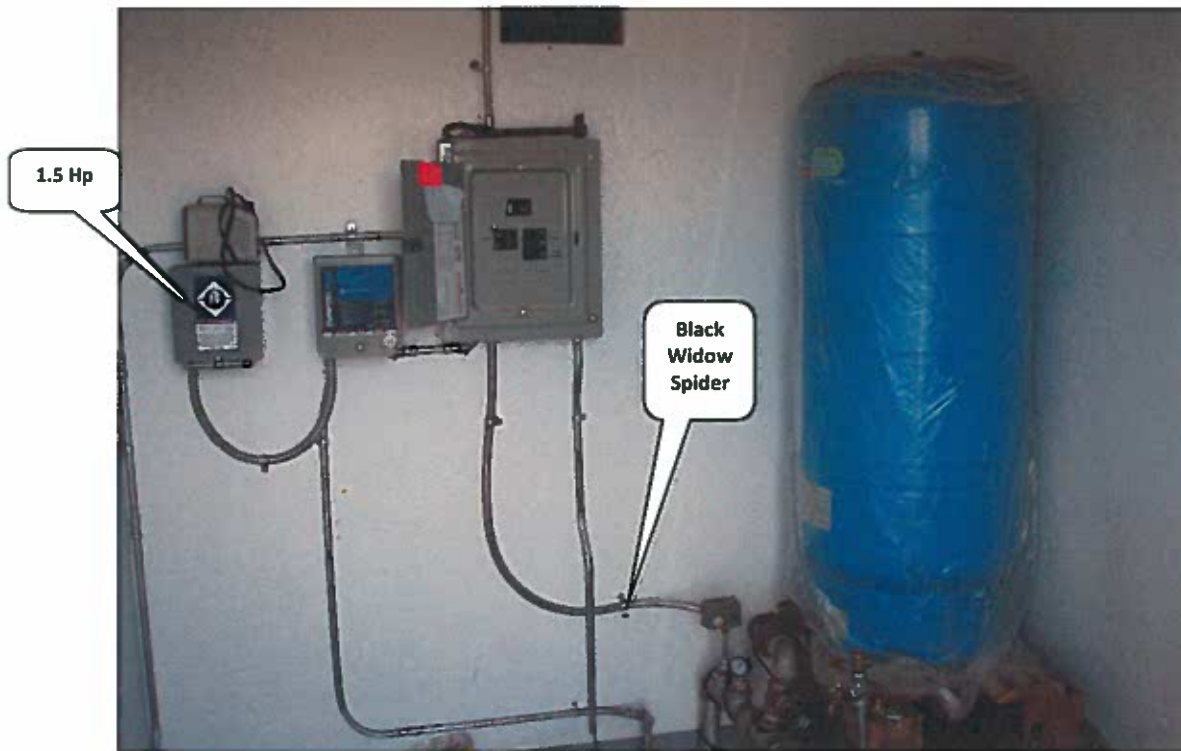
ABOVE: View inside of pump house with electrical box identifying pump as 1.5Hp
